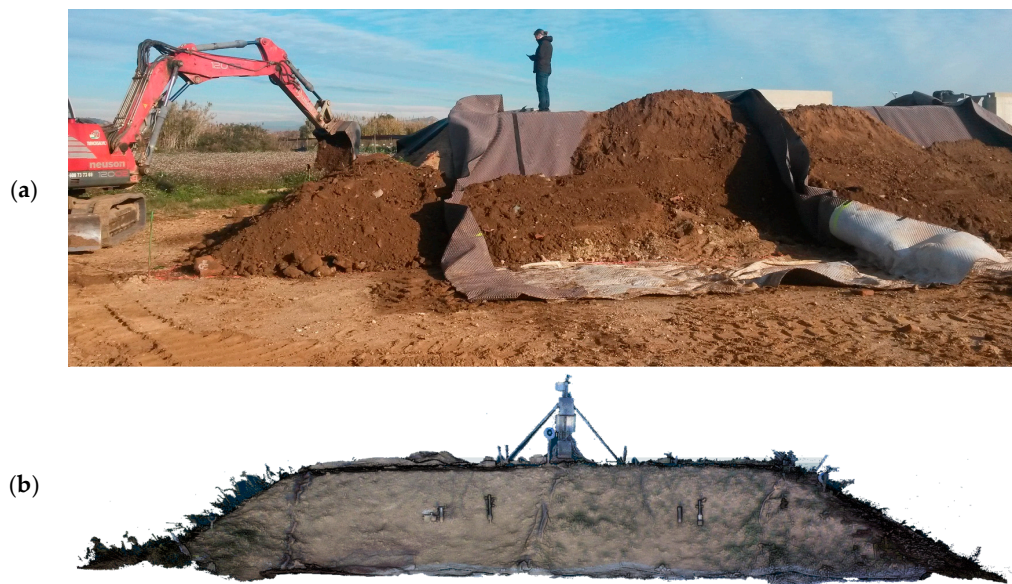
Figure 1. (a) Photograph of the embankment during the construction; (b) 3D view of the point cloud obtained by terrestrial laser scanning.
