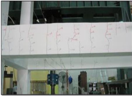
Figure-10. Vertical flexural cracks on the beam.
