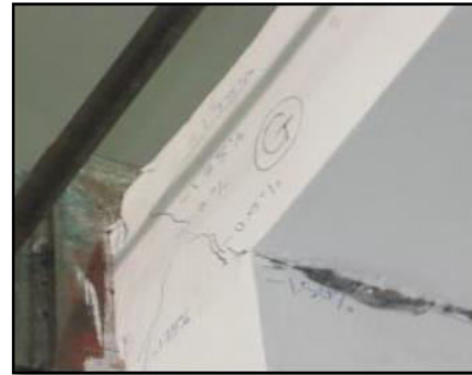
Figure-12. Diagonal cracks at corner joint.
