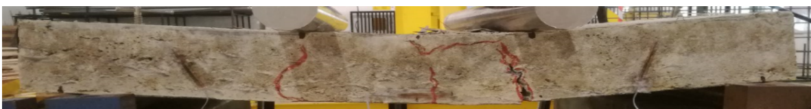
Figure 9. Cracking pattern at the failure of S1-1.
