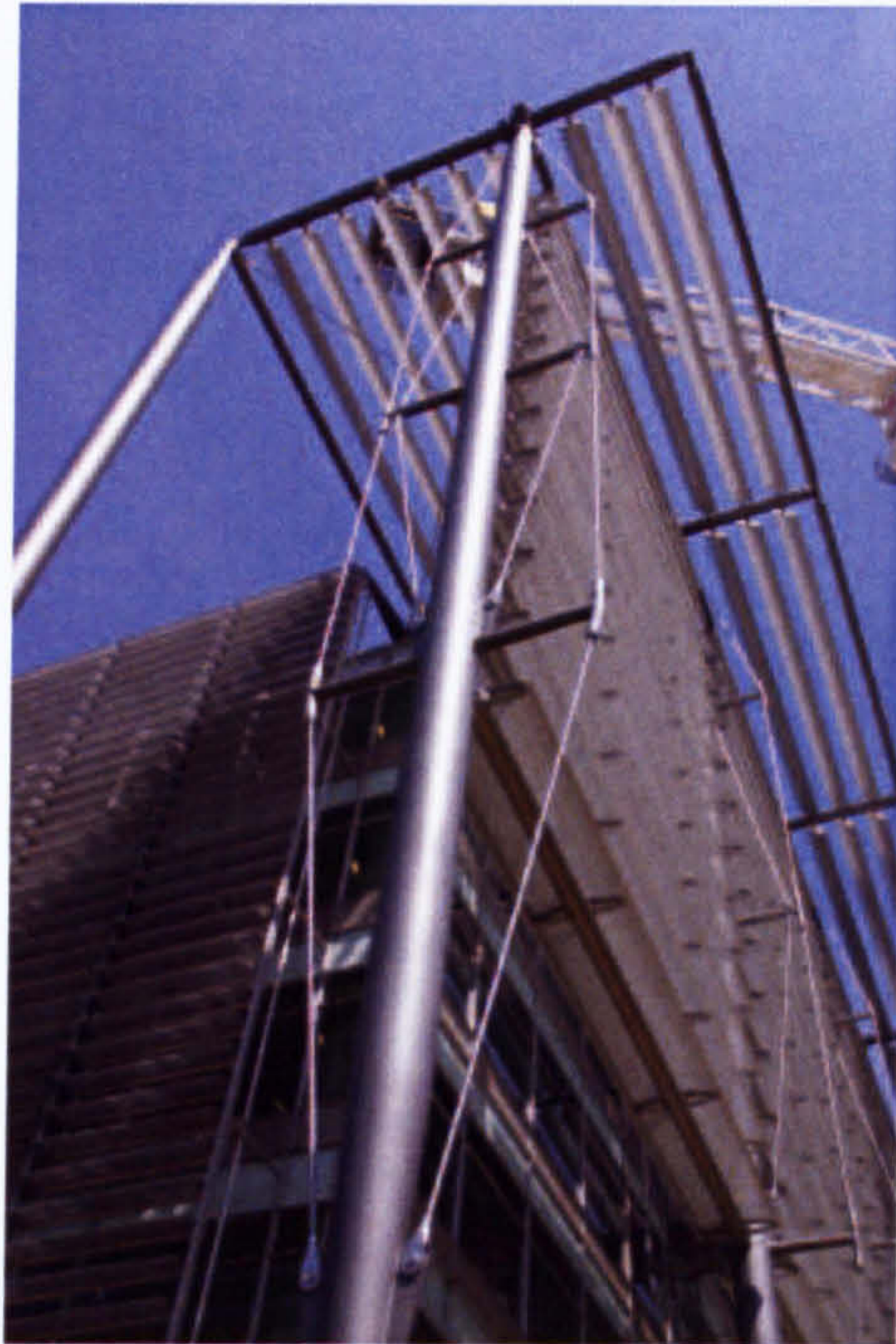
Figure 1.3: Building 5 at Chiswick Park, London—the stayed column system was adopted for the façade in conjunction with the shading fins.
