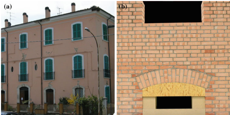
Fig. 1 Old URM building during the L'Aquila earthquake on April 6th, 2009, showing spandrel failure a and detail of a spandrel test unit ( b , Beyer and Dazio 2012a )
