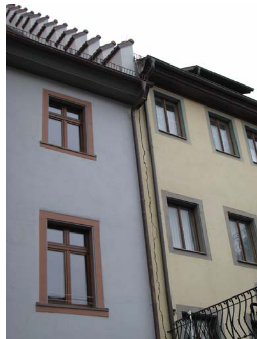
Fig. 3 Vertical open crack in the city centre that cuts two buildings from the ceiling to the roof
