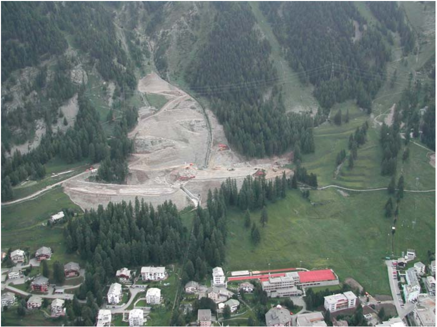
Figure 6. Combined avalanche/debris flow retention dam (under construction in 2003) protecting Pontresina at the foot of the Laviner Giandains gully. (Photograph: M. Hiller SLF).
