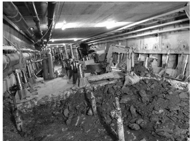
Fig. 1 Heave of the floor beneath the carriageway of the Chienberg Tunnel
