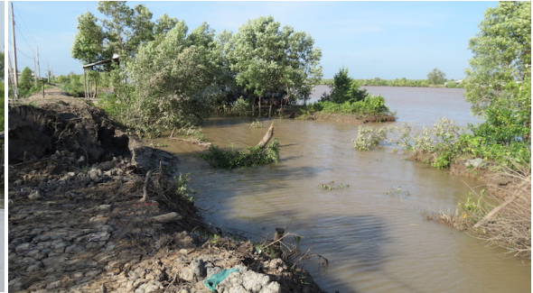
River bank breach/erosion
