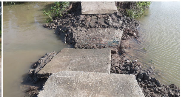
A collapsed path to a village in Tam Giang Dong Commune
