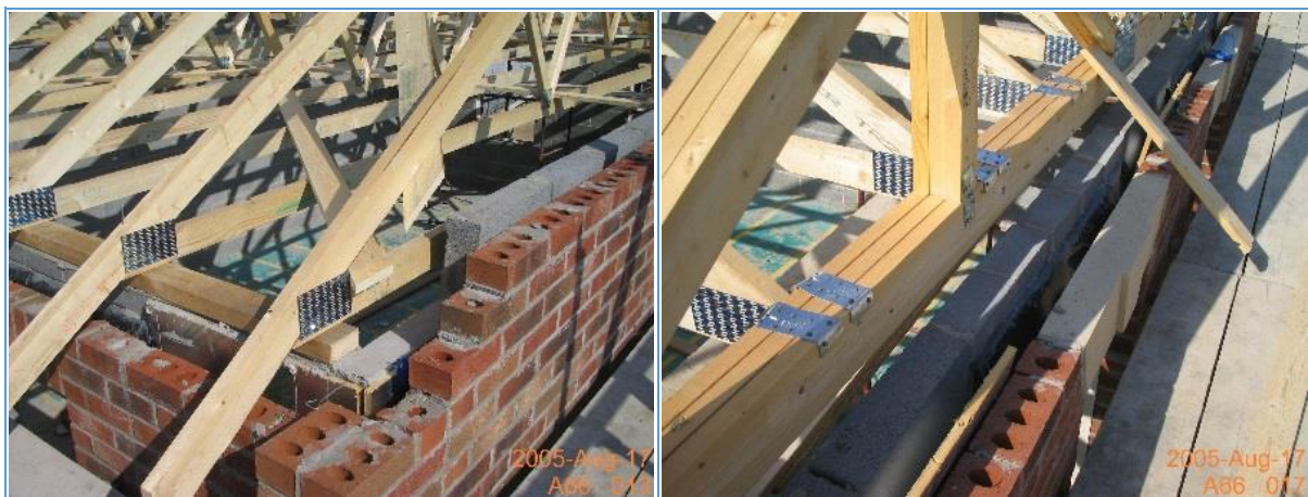
Figure 27 Issues with partial-fill boards at eaves, wall plates and top storey lintels
