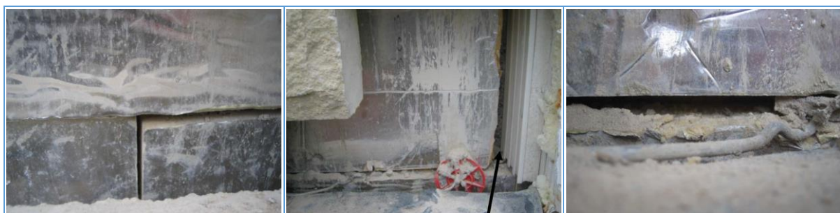
Figure 15 Deconstruction allowing gaps to be seen in the partial-fill insulation, from Wingfield et al., 2009.
