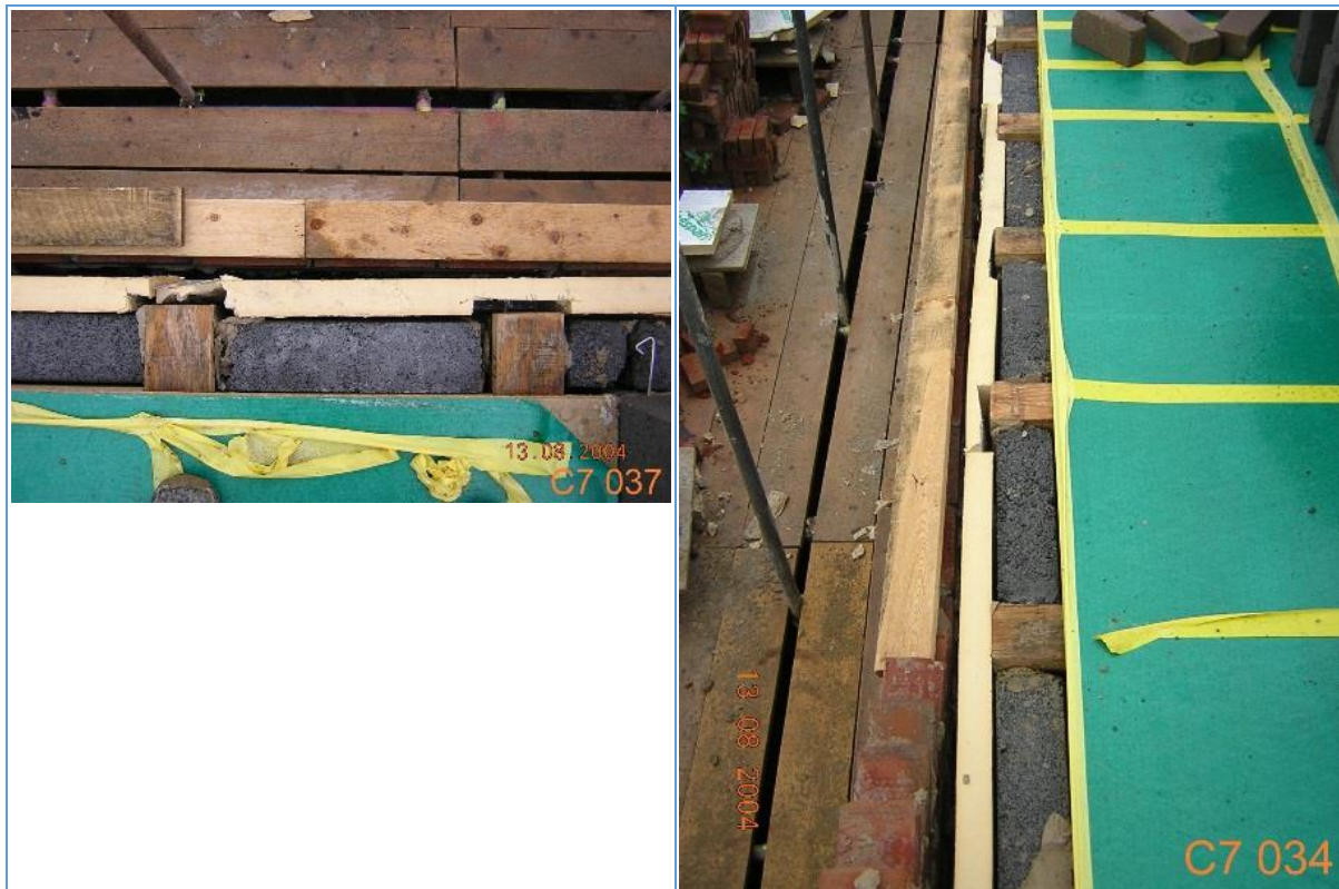
Figure 28 Missing/displaced insulation due to wall protrusions
