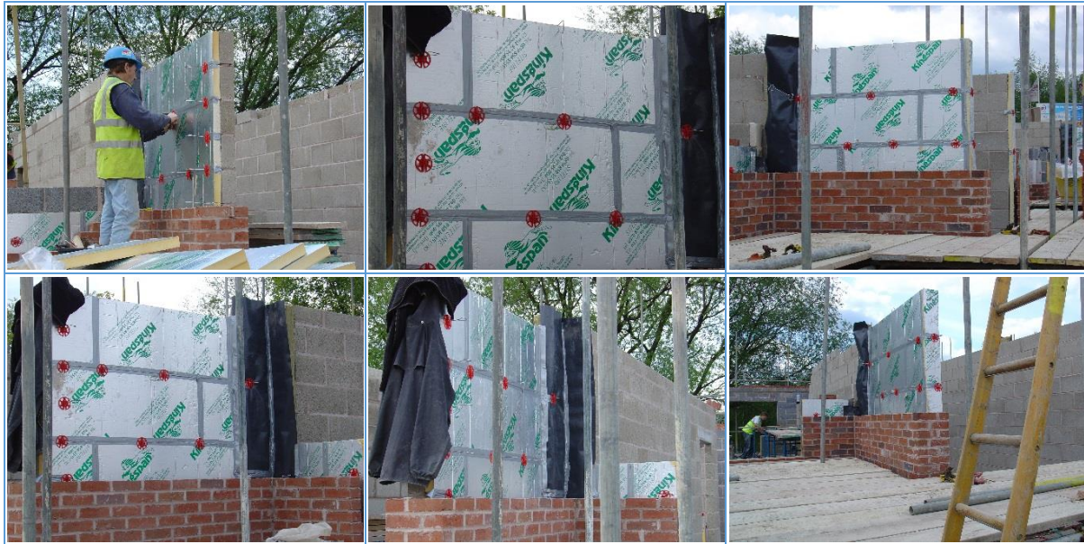
Figure 18 Partial-fill insulation being installed in standard brick-block masonry construction in an apartment block in Sheffield.
