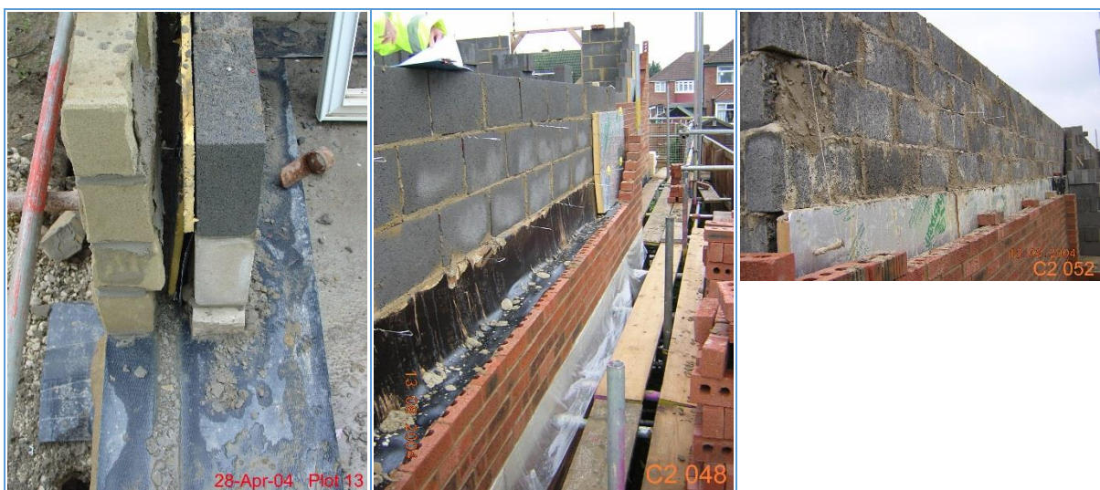
Figure 25 Issues with partial-fill insulation around cavity trays
