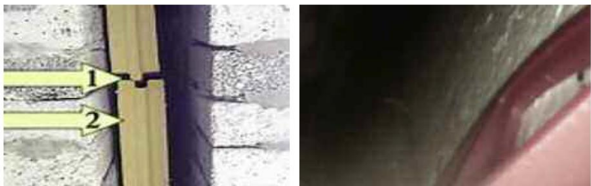
Where the board is poorly fitted (usually by a bricklayer) and gaps are present this allows cold air to circulate around the insulation
