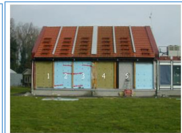
Figure 11 Partially filled test walls displaying lower than expected R-values compared to fully filled test walls (Hens et al., 2006)
