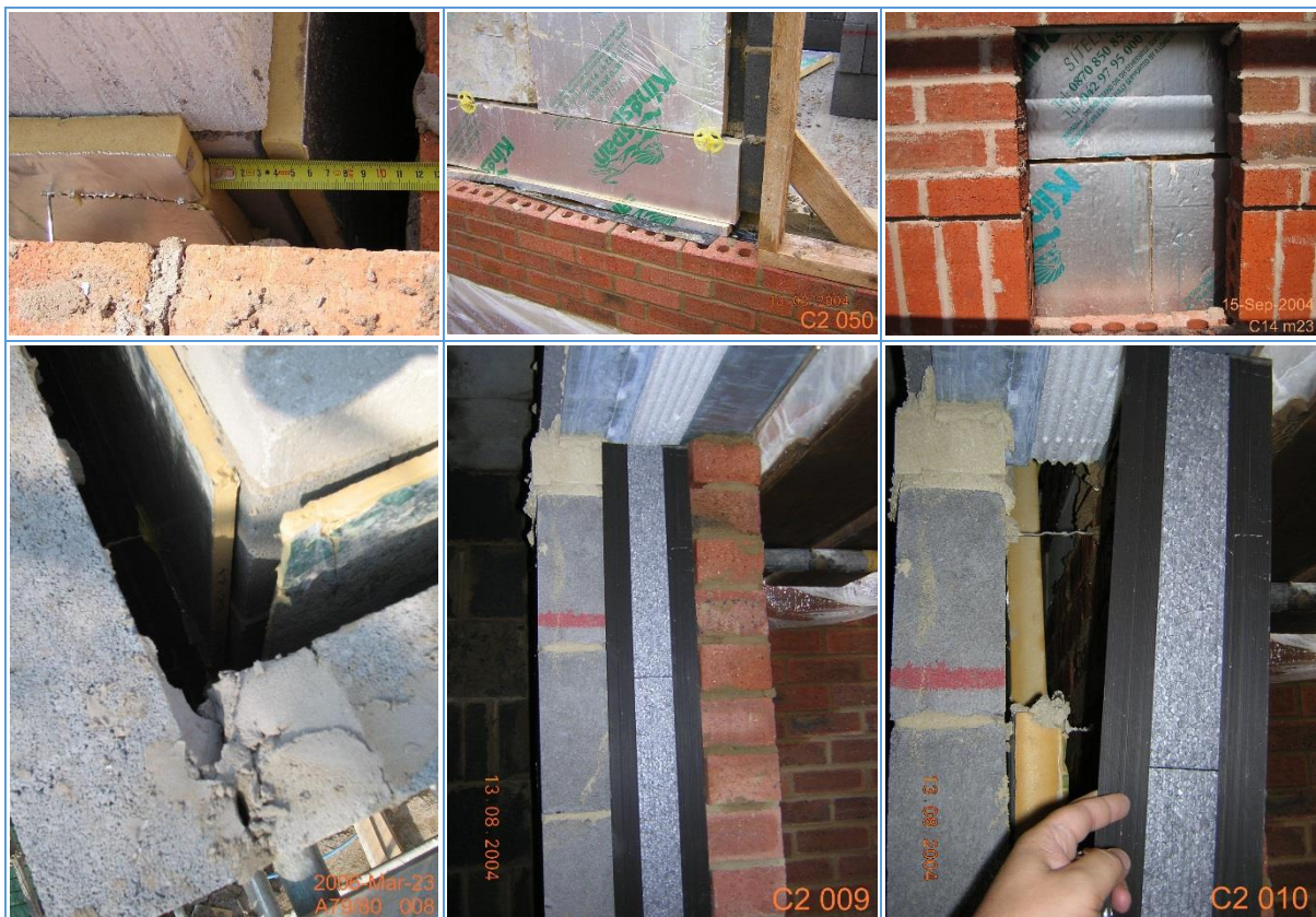
Figure 23 Gaps between and around partial-fill insulation boards
