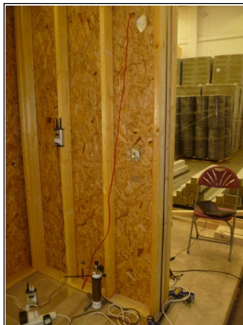
Figure 5 Tracer gas (CO 2 ) cylinder, regulator, solenoid valve and injection tube.
