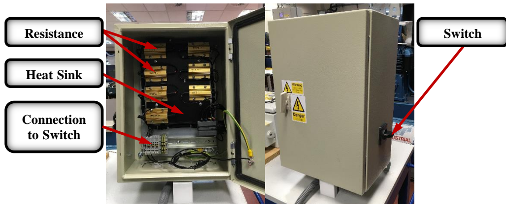
Figure 5.19 Photograph of external resistor bank
