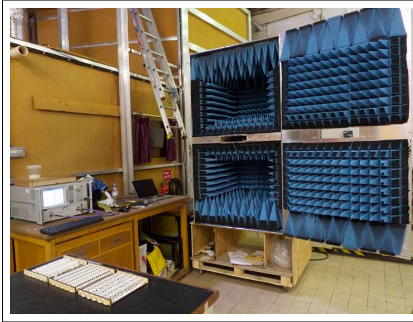
Completed anechoic chamber.
