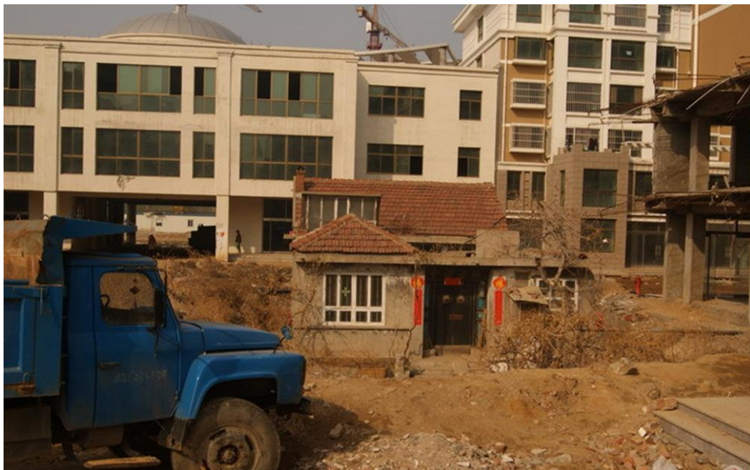
Picture 13 Wen Quan Tang Village Redevelopment Construction Going on While a Village House Sits in the Construction Site
