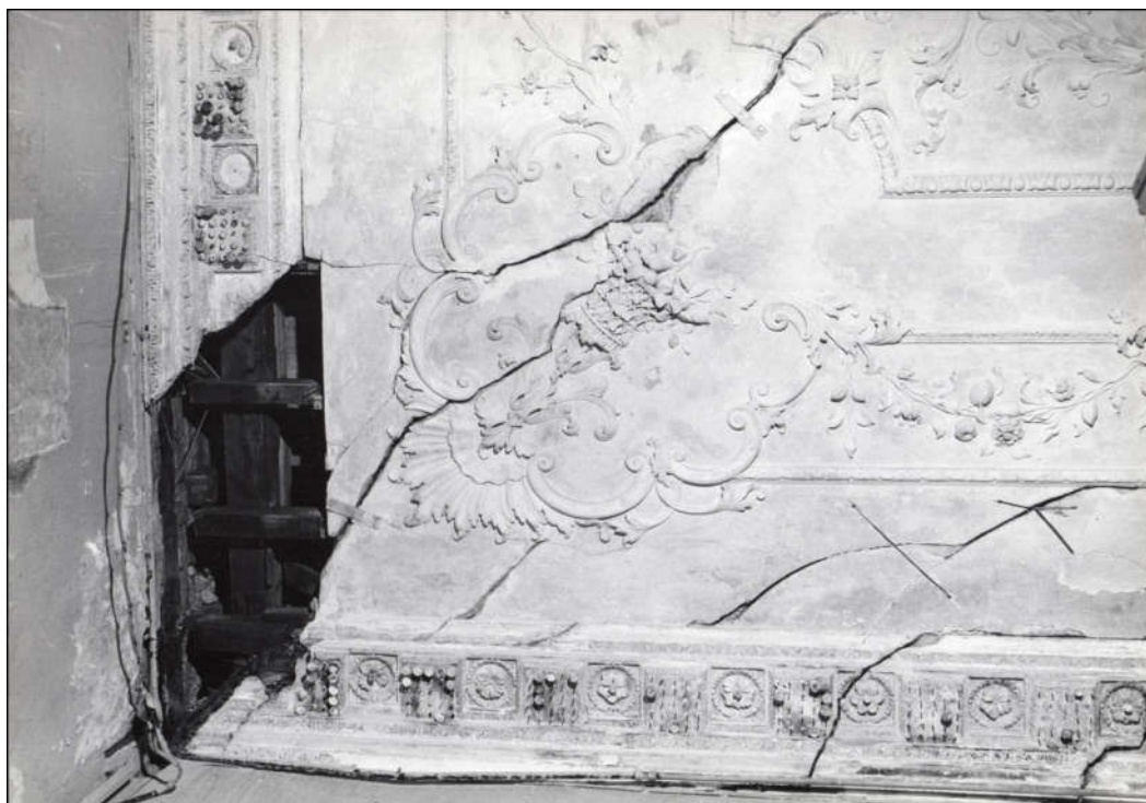
Figure 7.6. Damaged portion of the Dining Room ceiling. All the original decorative plasterwork shown here was re-used when the ceiling was repaired and reinstated. (Fairfax House Archive.)
