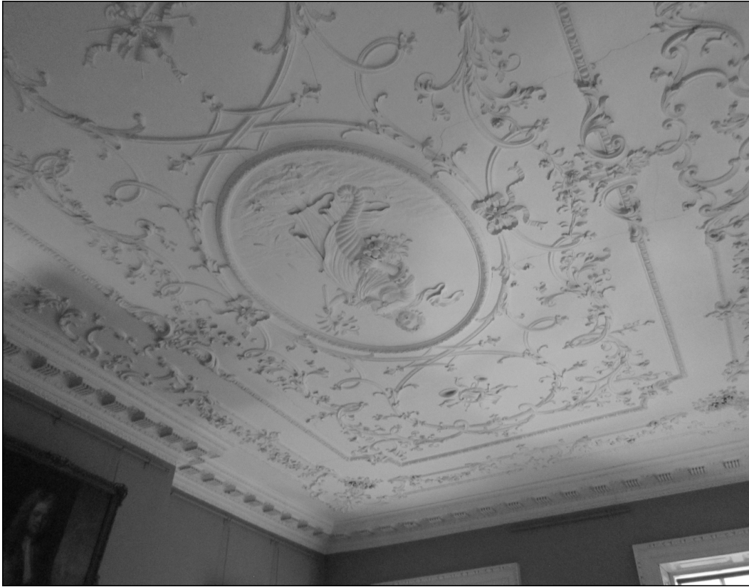
Figure 1.17. The Dining Room ceiling. The figure in the central oval represents ‘abundance’. (Author’s photograph, 2014.)
