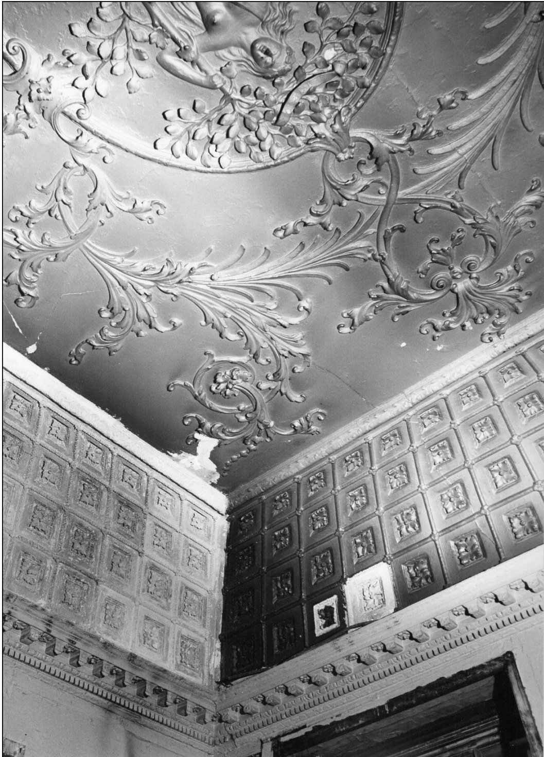
Figure 7.4. Cleaning and repair of the plasterwork coving and ceiling in the south-eastern corner of the Drawing Room during the restoration of the house in 1983. The portion of coving on the left has had its covering of modern paint removed and has been cleaned down to the original plaster. On the section of coving to the right removal of the paint section by section is just beginning. The ceiling is still covered in modern paint awaiting removal, but the good quality of the original plasterwork under the paint can clearly be seen despite the blocking up of much fine detail. (Fairfax House Archive.)
