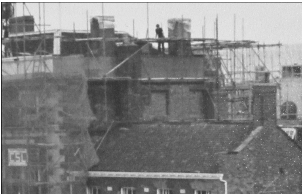
Figure 1.8. Detail of a photograph of the south-eastern end wall of Fairfax House taken during the restoration of 1983-84, undated but probably late summer 1983, showing two rearmost window embrasures infilled with new brickwork. (Fairfax House Archives.)
