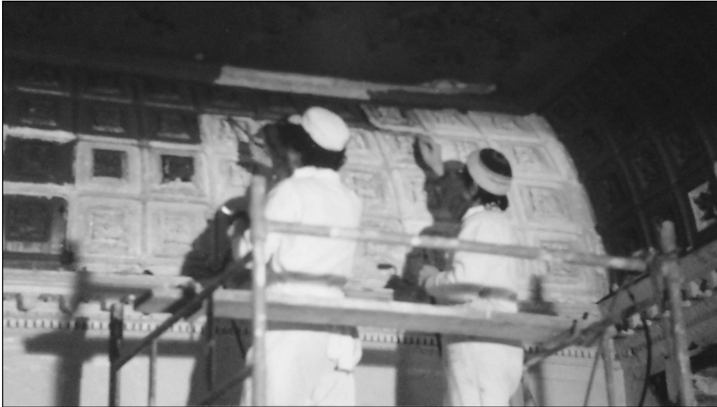
Figure 7.5. Photograph taken in the summer of 1983 of the removal of the red paint applied by the cinema company from the Drawing Room ceiling. All this work was done by hand by employees of the York decorating firm Bellerby's. (Fairfax House Archive.)
