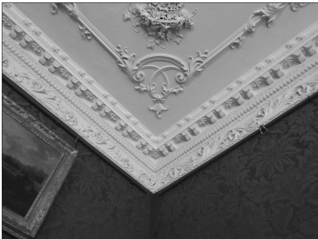
Figure 1.23. Detail of the Saloon ceiling, showing cornice decoration and frieze. Above each modillion is a lion mask. (Author's photograph, 2017.)
