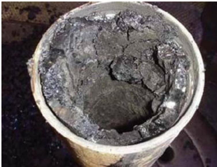
Figure 1.1. Asphaltenes clogging a pipe. Courtesy of A. Pomerantz, Schlumberger [20].
