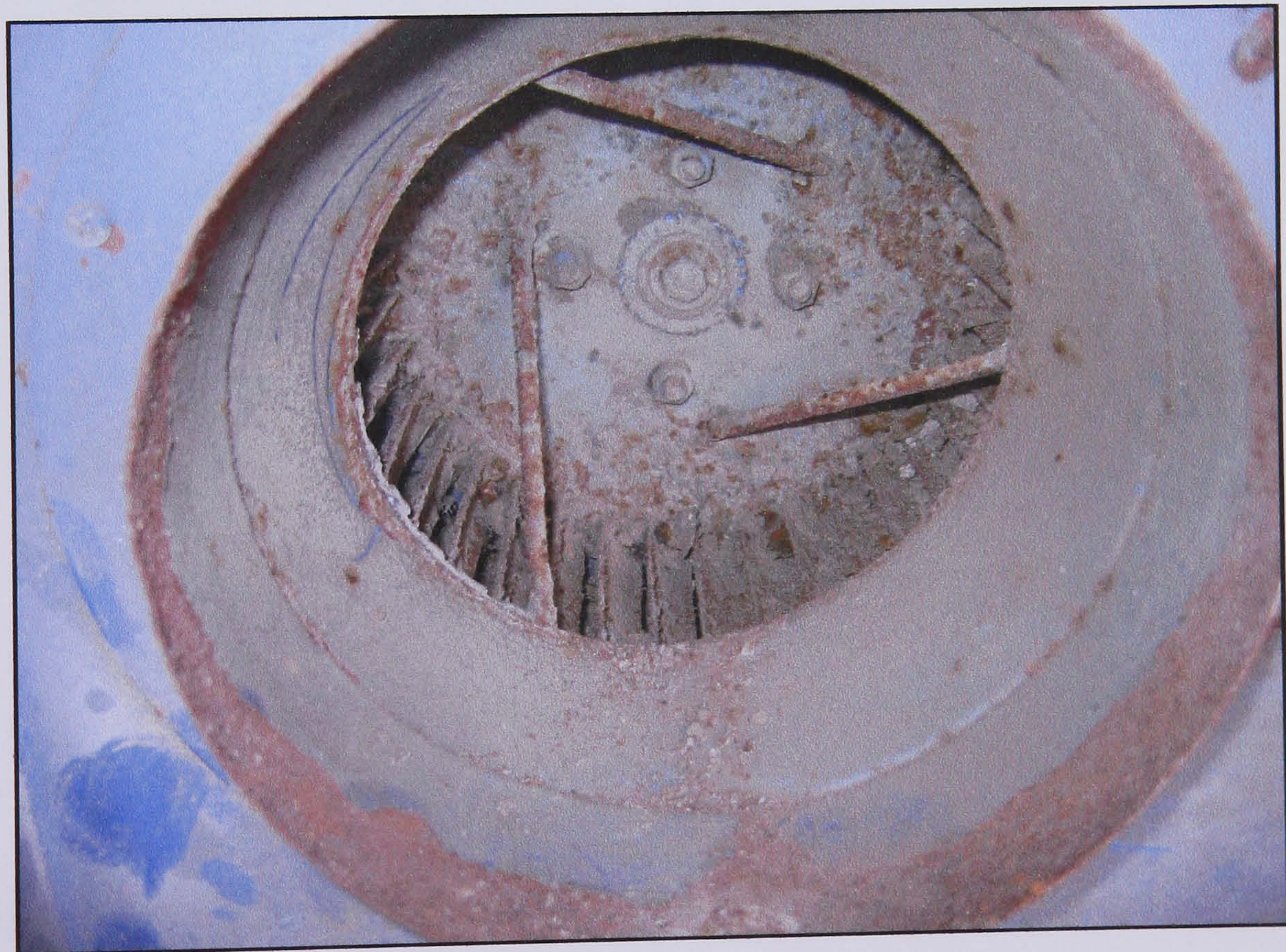
Figure 2-8: Poor maintenance of a mechanical ventilation system
