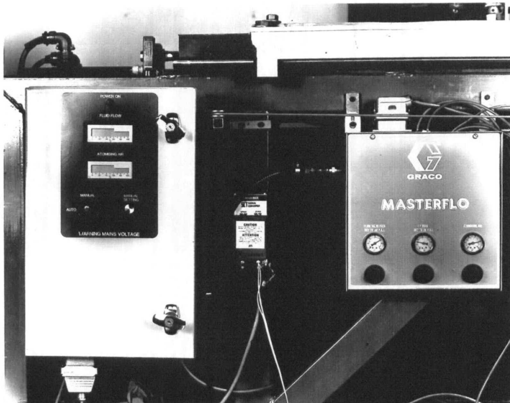
Figure 4.4: Master-Flo pneumatic actuated controller.
