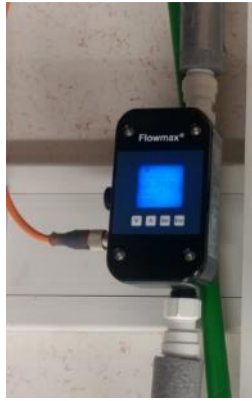
Figure 3.6 Water Flow Meter
