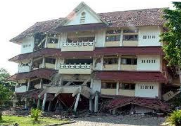
Government office damage from Bantul earthquake
