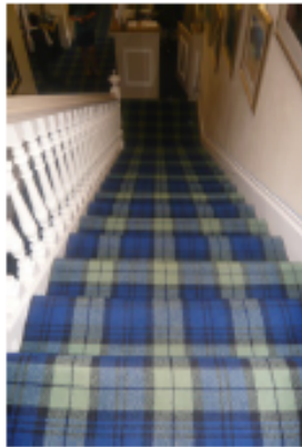
Image 1: Patterned carpet obscuring stair edges
