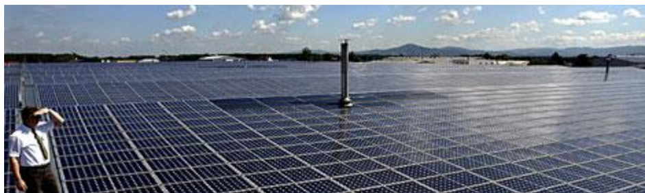
Figure 1-2 A massive array of single crystal silicon solar cells, covering 40,000 m 2 of a warehouse rooftop in Buerstadt, Germany. The plant is capable of delivering approximately 5 MW of power. [Reuters file photo]
