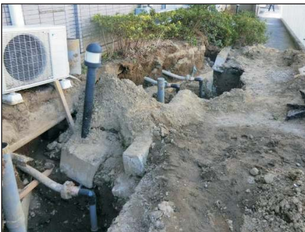
Figure 17. Settlements of the ground around buildings with deep foundations in Katori city.
