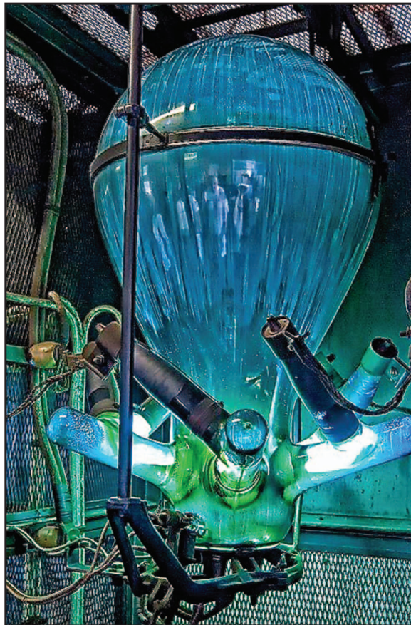
FIGURE 2 – A multinode mercury-arc rectifier still in operation in October 2010 at Manx Electric Railway substation at the Laxey Isle of Man. (Image courtesy of Tony S. at Talk Electrician Forum.)
