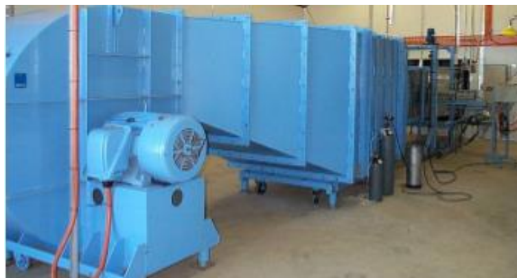
Figure 1.2. Main, rear fan for University of Queensland Wind Tunnel.
