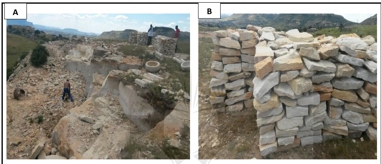
Figure 7: Artisanal mining of sandstone using chisel and hammers. (A) Mining area on the mountain; (B) stockpile of sandstone
