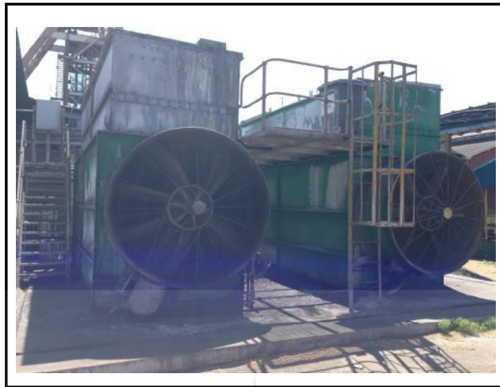
Figure 45: Cooling tower fan
