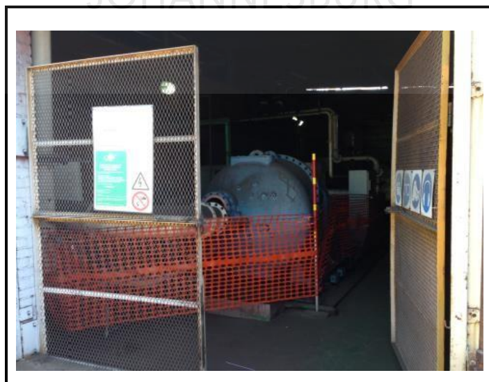
Figure 44: Compressor at the shaft
