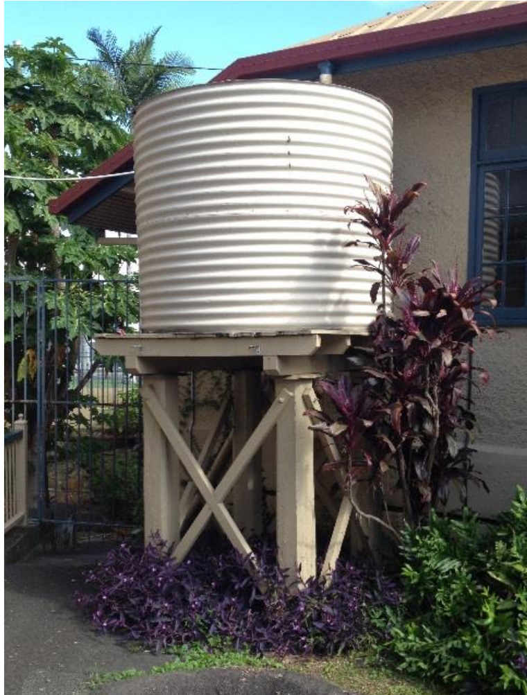
Figure 6. Historical design of a rainwater tank made of galvanized iron where water is gravity-fed from a tank stand.
