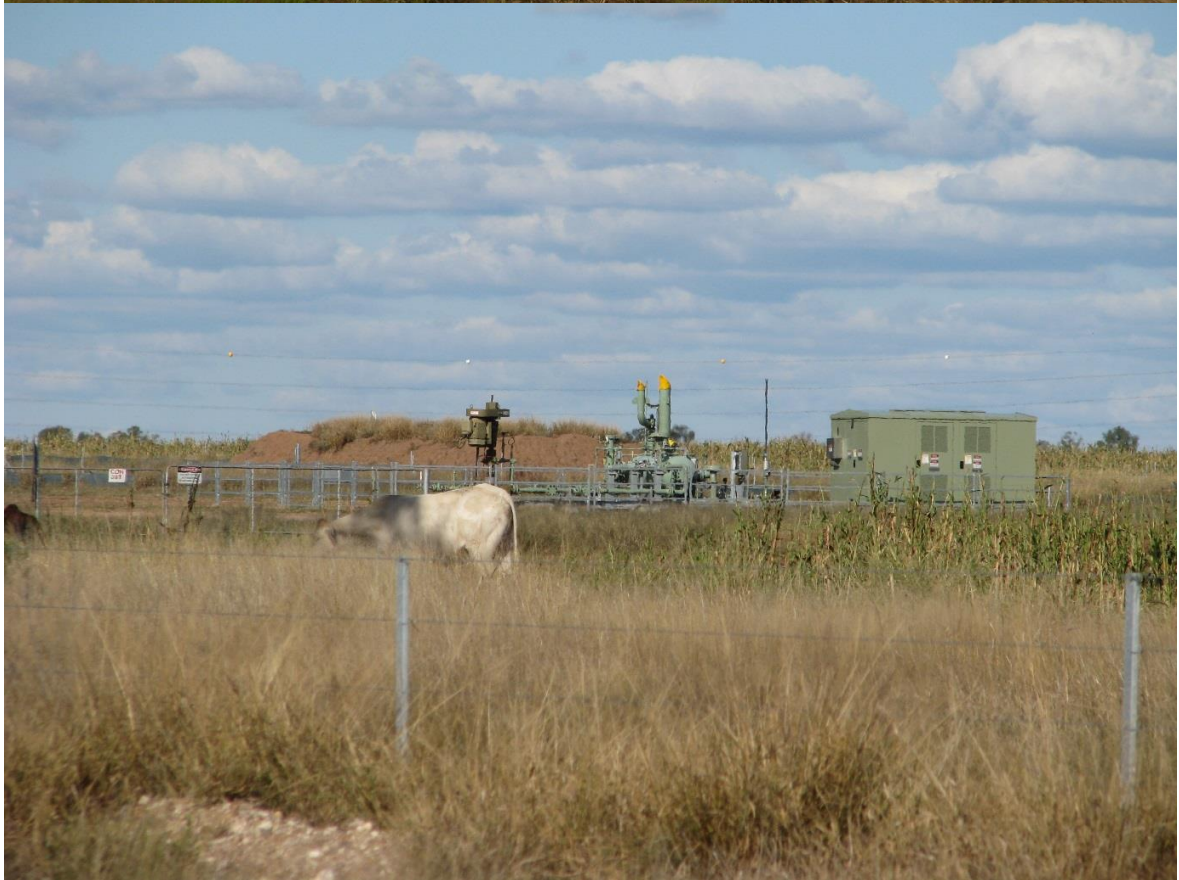
Image 29 Parts of a CSG well (top) and an operating CSG well near Miles (bottom) (source: author 2015)
