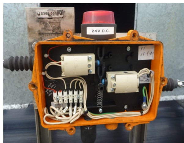
FIGURE 13. SIF#1 – A100 - safety switch.
