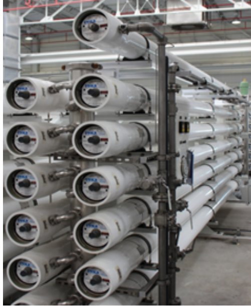
Figure 11. Spiral wound RO membranes installed in Groundwater Replenishment System (GWRS) Advanced Water Purification Facility (Fountain Valley, California), taken at the Orange County Water District.
