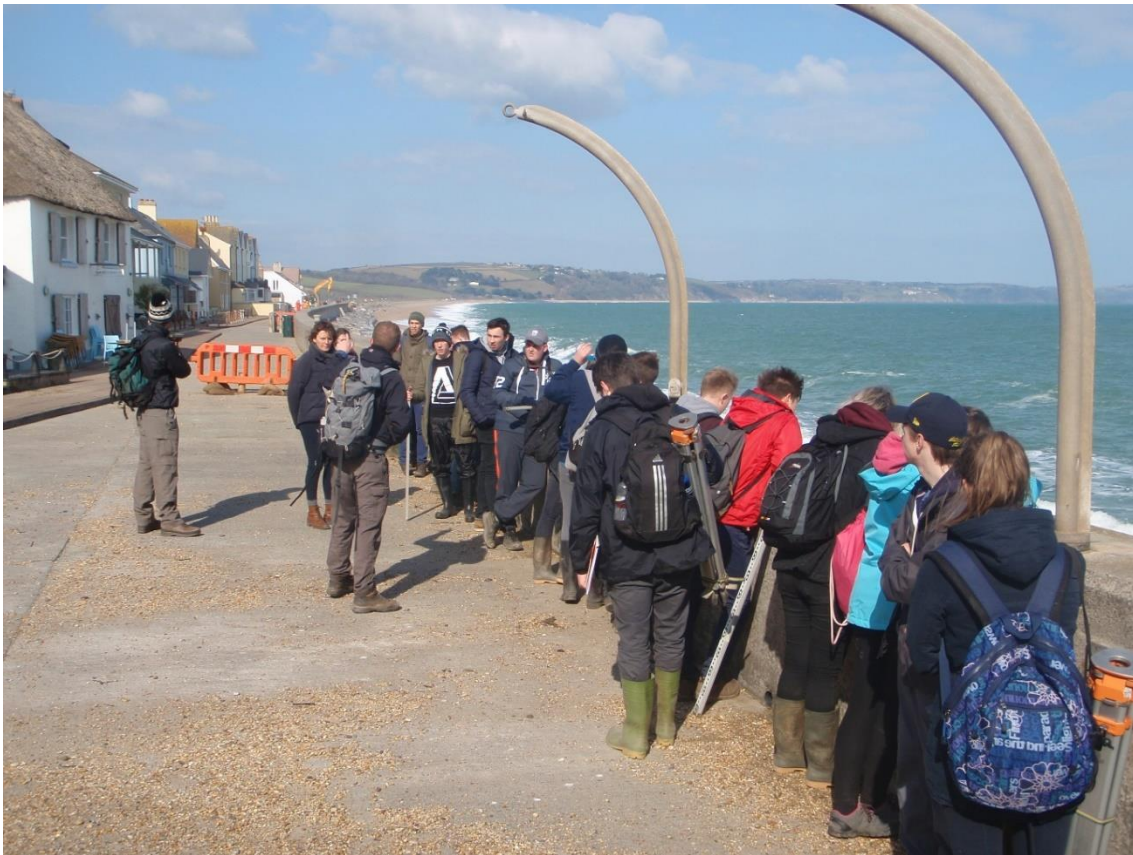
Photo 5.2 A tutor talks about storm damage to the sea wall at Torcross (Slapton, Group G, author photo).
