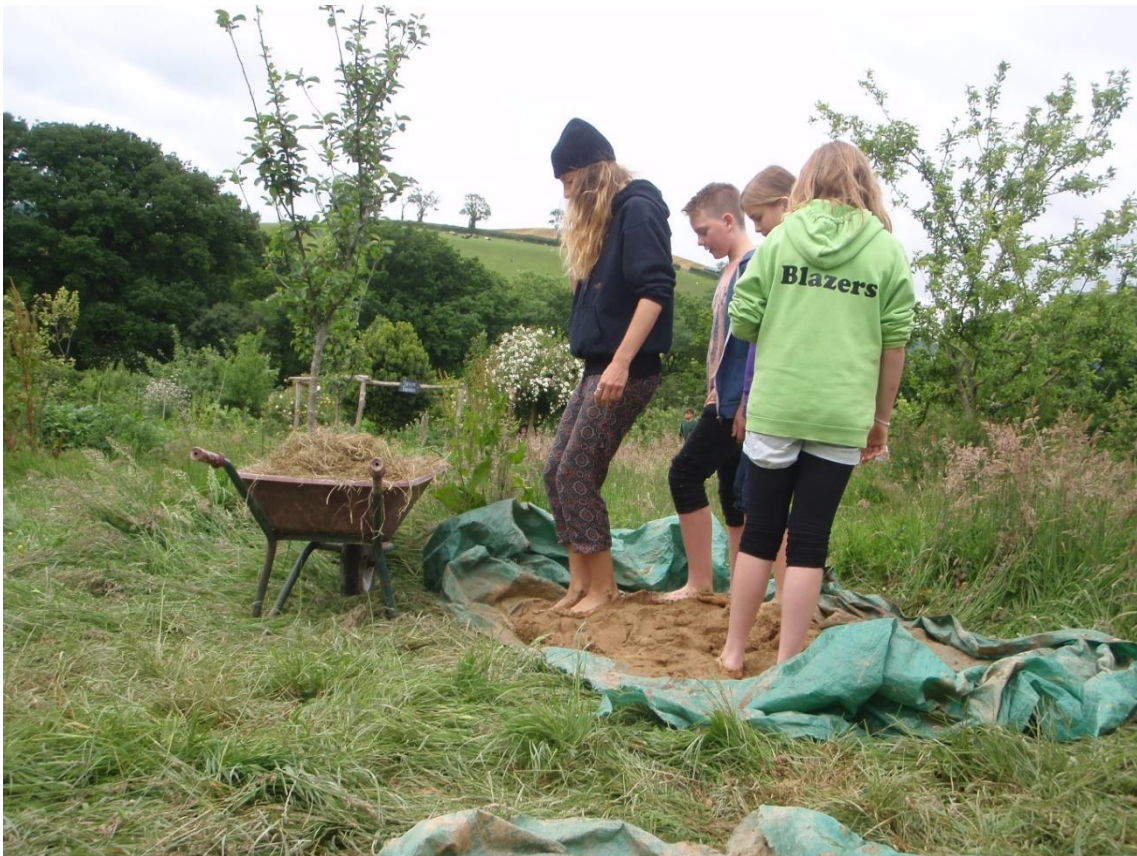
Photo 5.3 Students puddle clay mixed with sand and hay with their feet, to make cob mixture for construction of the lime kiln (author photo).
