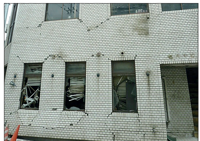
Figure 4. Tsunami-preceding seismic damage indicated by conjugate shear cracking of a building facade in Kamaishi
