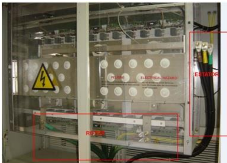
Figure 88 Photograph of compartments A and B. The photograph is courtesy of INDRA.
