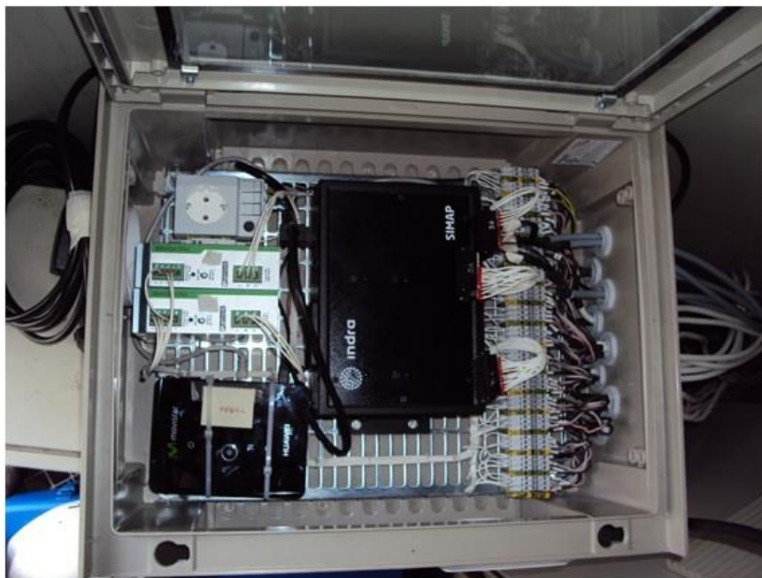
Figure 93 Data acquisition cabinet of the INDRA RCM system installed in one of the ACCIONA 1.5 MW wind turbines. The photograph is courtesy of INDRA.
