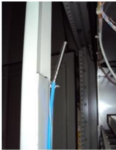
Figure 105 Temperature sensor. The photograph is courtesy of INDRA.
