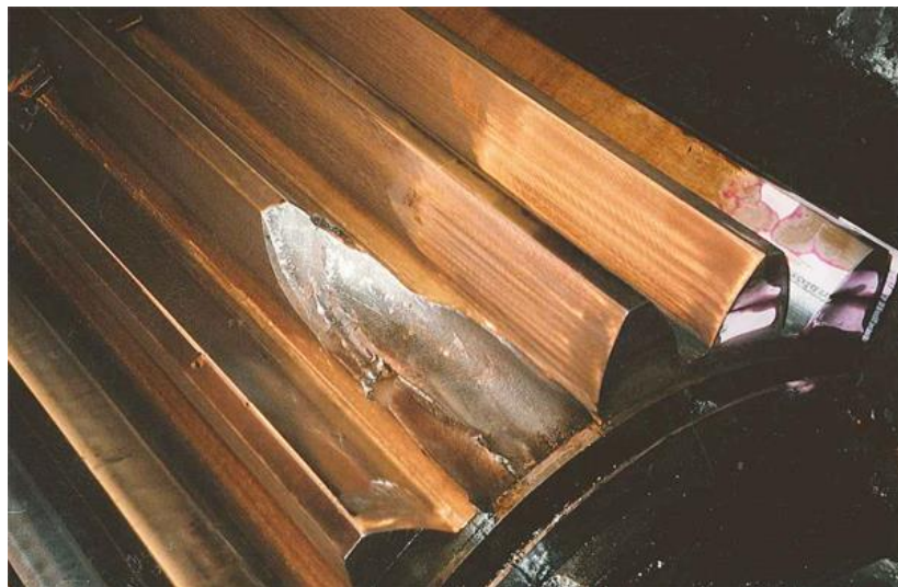
Figure 30 broken teeth related to unanticipated wear of bearing/pinion [92].
