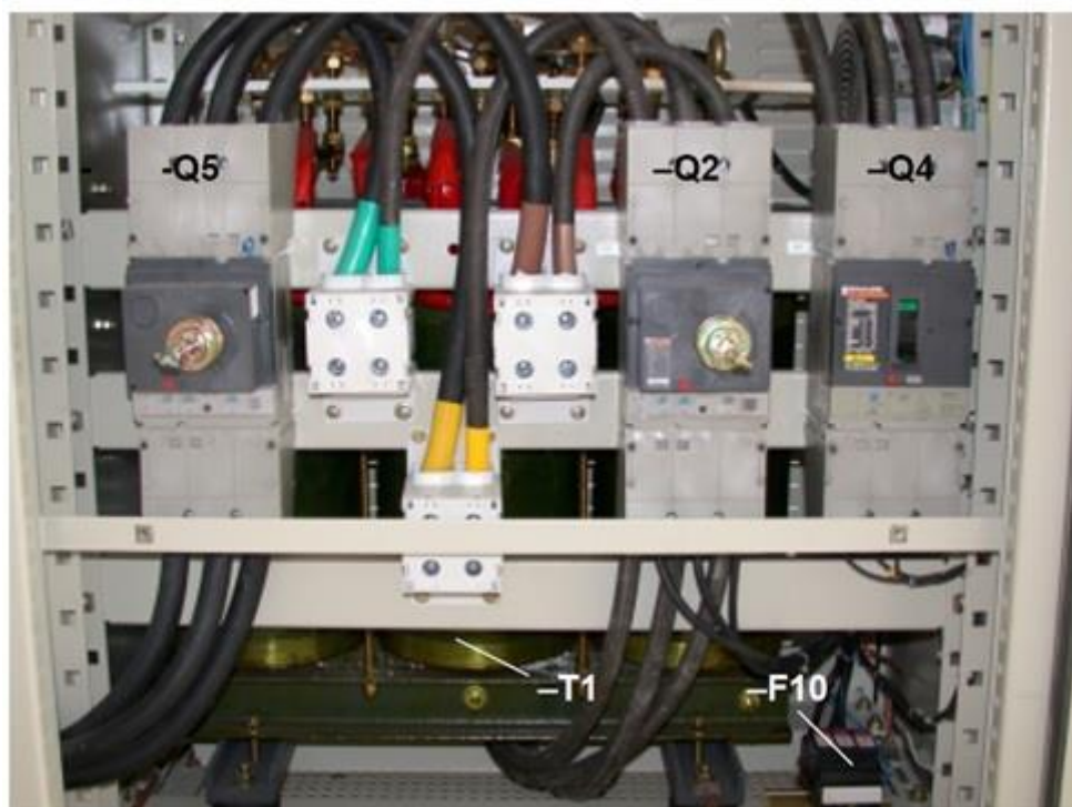
Figure 92 Photograph of compartment G. The photograph is courtesy of INDRA.
