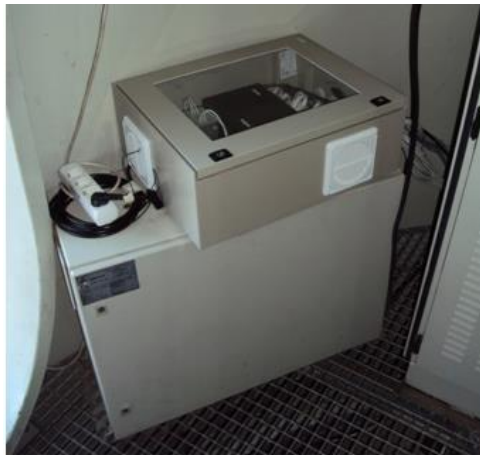
Figure 99 INDRA data acquisition unit. The photograph is courtesy of INDRA.
