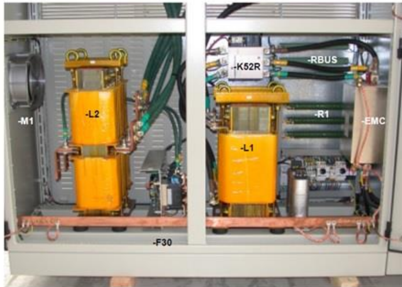
Figure 89 Photograph of compartments C and D. The photograph is courtesy of INDRA.
