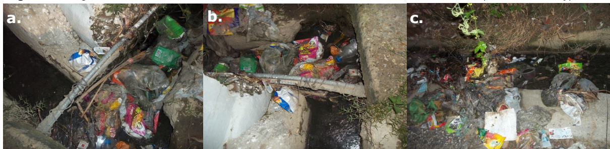
Fig. 3 (a-c). Water supply pipes passing through drains at the old Jammu distribution point.
