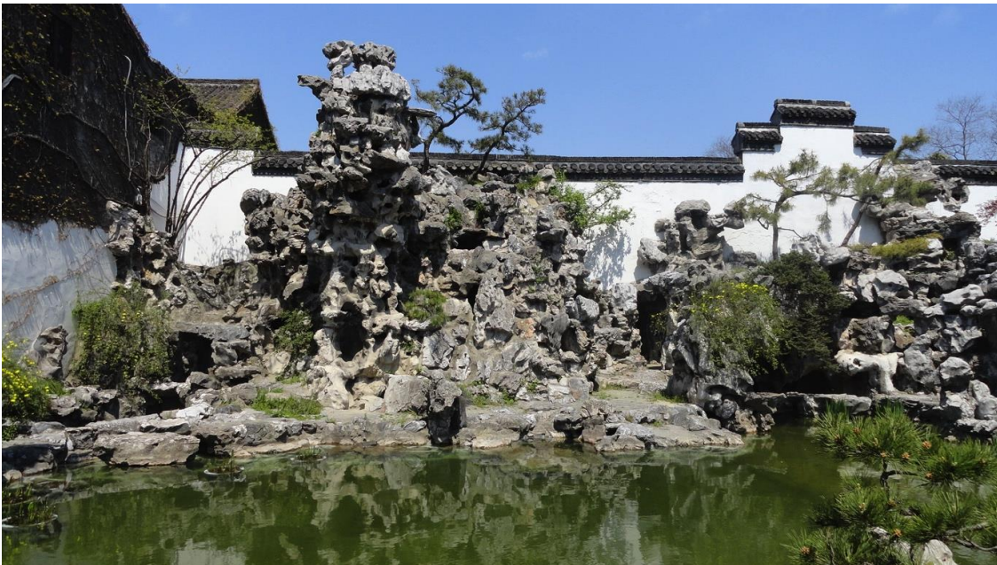
Figure 6-16. Current northwest side of the rockwork, where the rockwork has been repointed and large trees have been removed. (Source: author, 2013.)
