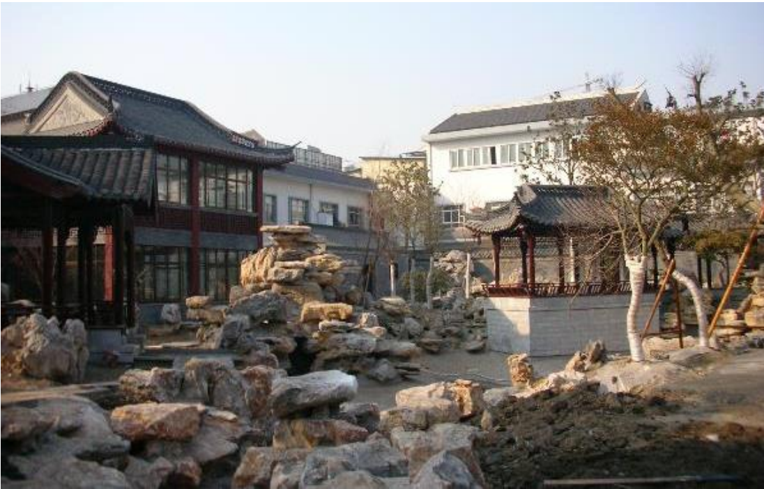
Figure 4-19. The extended part under construction, which shows that a large quantity of rockwork was constructed around buildings. (Source: author, 2013.)
