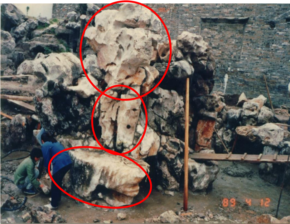
Figure 6-15. Newly constructed rockwork added to the east side of the rockwork. Comparing them with the size of people working on site, it is clear that the rocks used for restoration are about one metre long or longer. Photo taken in 1989. (Source: Administration Office of He Garden, 'Resume of Buildings in He Garden (Resume of the Conservation of the Rockwork in the Mountain House of Sliced Stones)', held by the Administration Office of He Garden)
