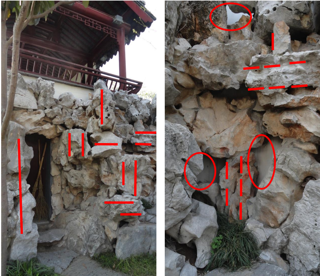
Figure 5-20. Rockworks in the north expansion part. Red circles show the gaps between rocks, where the wall is exposed; red lines shows the patterns of rocks, which indicated that vertical and horizontal patterns are mixed together in an irregular way. (Source: author, 2013.)
