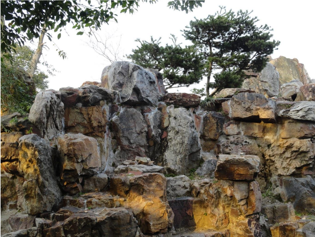
Figure 8-12. Rockwork under reinforcement in Swallow Garden, in which the repointed gaps between rocks are nearly invisible. (Source: author, 2017.)
