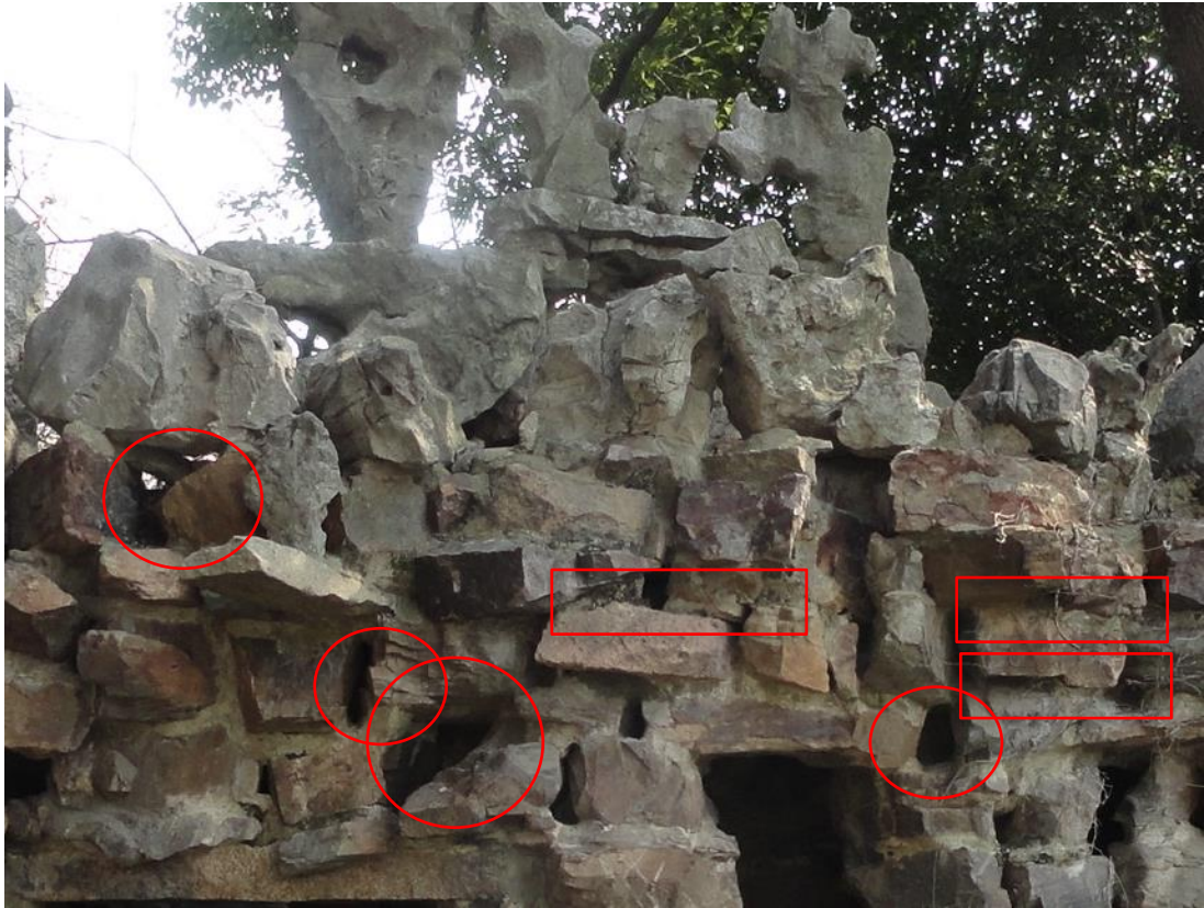
Figure 8-1. Remaining historic rockwork in the Garden of Fuzzy Boundary. The circular frame shows the gaps that were intentionally created; the rectangular frame shows the original joints. Small gaps between rocks in the original historical rockwork in Garden of Fuzzy Boundary ( Xukuo yuan 虚廓园), Changshu. (Source: author, 2013.)
