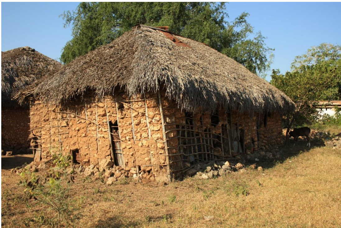
Figure 3.2: Derelict modern wattle-and-daub structure at Kilwa Kisiwani. Note coral rag bound into daub matrix, and concentration of coral pieces as a result of wall collapse, creating potential magnetic anomaly. Photo by author (2013)
