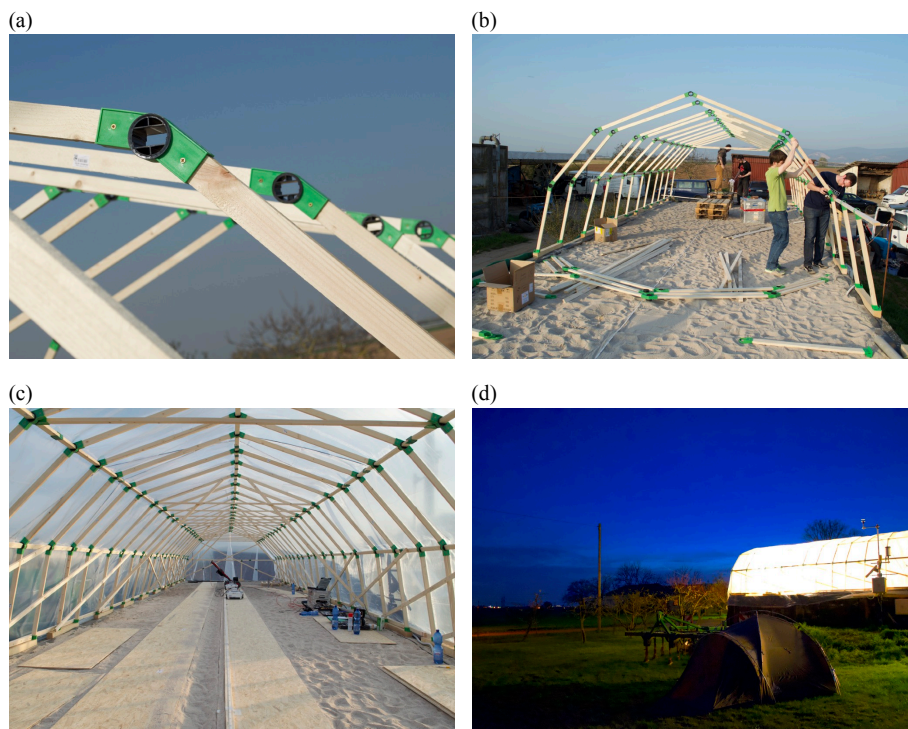
Figure A.1 (a) In order to construct the roof at ASSESS, VarioQuick® elements were used to connect roof battens. (b) The erection of the roof required many helping hands. (c) The roof allowed for long-term fluctuating groundwater table and infiltration experiments, that required continuous measurements for several days and (d) some camping at ASSESS.
