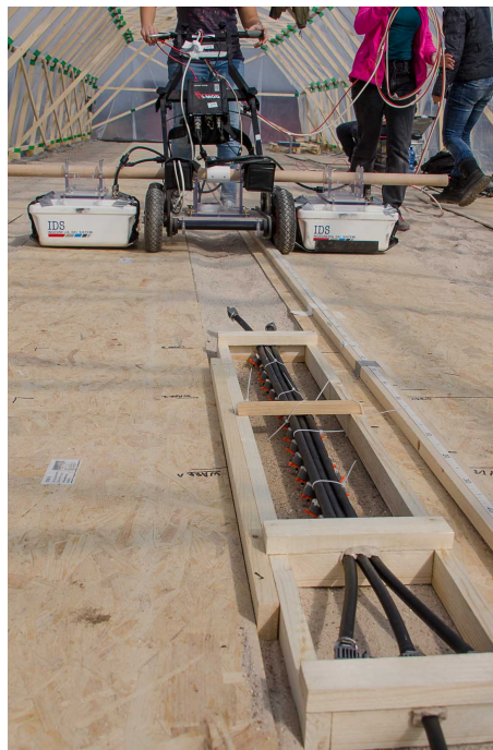
Figure A.2 The construction of a roof over ASSESS (Fig. A.1 ) allowed for long-term infiltration experiments. Hence, an infiltration device was created. The successful application of the prototype shown in this figure lead to a more advanced version (Fig. A.3 ). [from Klenk et al. (2015b) ]
