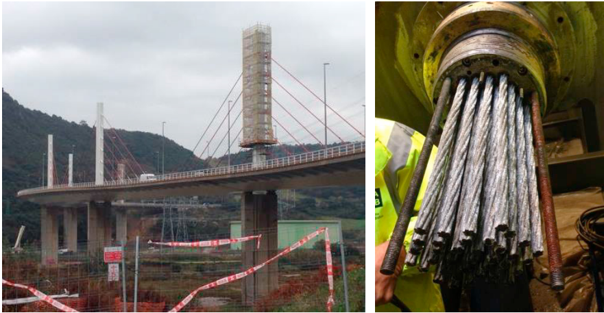
Fig. 2. Left: Bridge during inspection tasks; right: strands conforming one of the bridge's tendons during an inspection.
