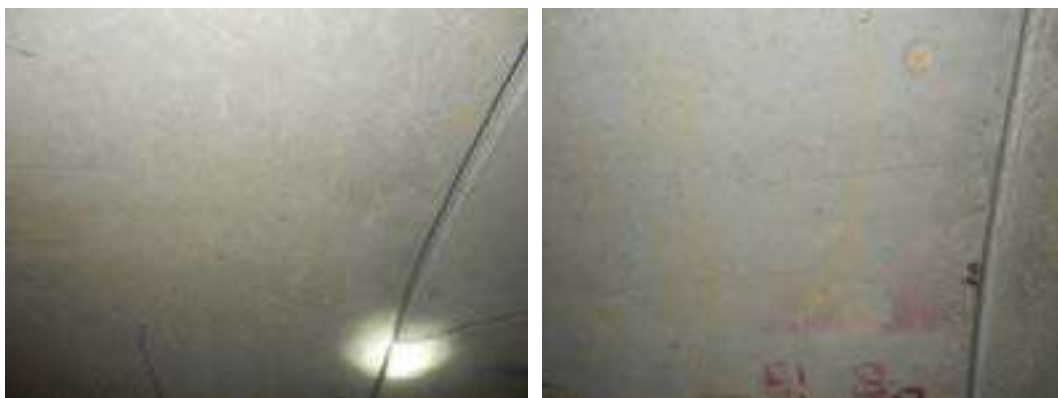
Figure 1. Sub-horizontal cracks at the sides of the tunnel. Misaligned segments.
