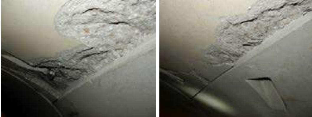
Figure 2. Concrete detachments in the upper part of the lining ring.
