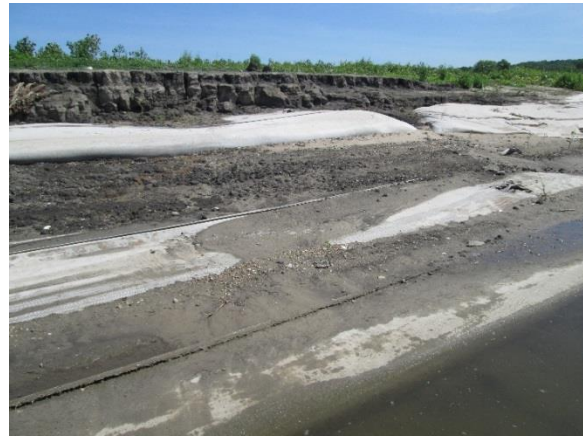
Figure 72. Sediment forming the artificial island in Lower Peoria Lake is eroded when waves overtop the torn or flattened geotextile tubes.
