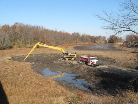
Figure 64. A long stick excavator removes sediment from temporarily drained Walton Lake at Litchfield, Ill.
