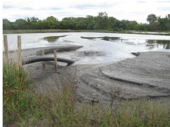
Figure 15. Sand and gravel settles out near the pipe at Fox Waterway Agency setting basin.
