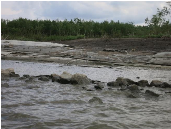
Figure 71. On Lower Peoria Lake geotextile tubes lose material after being torn. Protective riprap is in the foreground.
