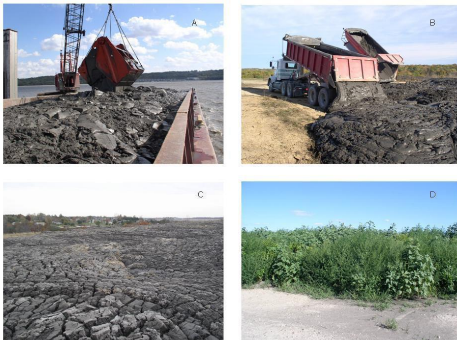
Figure C2. Sediment application as a topsoil substitute at Pekin, Ill., Landfill: A, clam shell bucket loading Peoria Lake sediment onto a deck barge; B, stockpiling sediment on top of Pekin Landfill clay cap; C, drying sediment one month after placement; D, volunteer vegetation thriving on sediment, unvegetated foreground is landfill clay cap, one year later.
