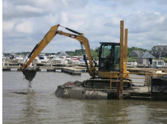
Figure 25. East Port Marina material is placed in a hopper in front of the excavator on the dredge. The displacement pump is below the deck.
