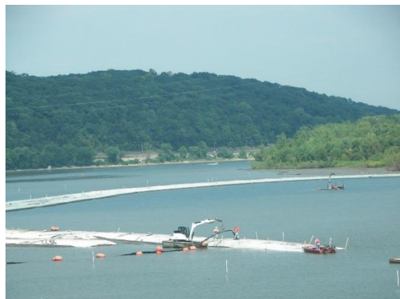
Figure 29. Material is pumped into geotextile tubes forming a ring that was later filled with sediment to form the island.
