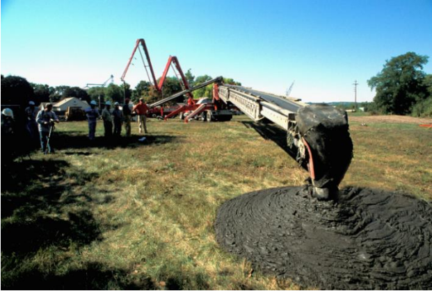
Figure 30. A truck-mounted telebelt typically used to convey concrete demonstrates its ability to handle wet sediment.
