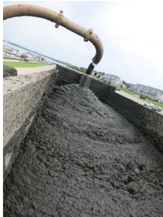
Figure 61. The Dry Dredge™ directly loads sediment from the river into trucks for placement at various locations.
