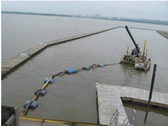
Figure 60. The Dry Dredge™ operating at East Port Marina. Sediment is forced through the pipe by a displacement pump.
