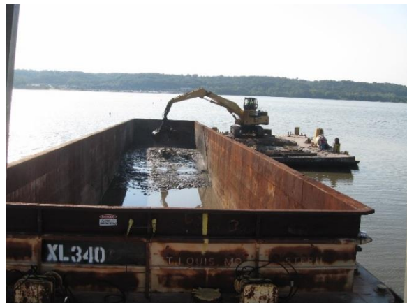
Figure 17. Excessive water in a barge where the hydraulic bucket is not draining adequately prior to placing sediment.
