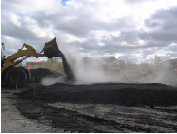
Figure 75. Dry biosolids are dumped from a front loader to be mixed with dried sediment.
