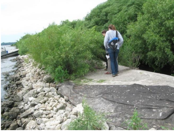
Figure 69. Students stand on a geotextile tube protecting an artificial island from waves at FWA. Riprap protects the tubes from ice and debris.
