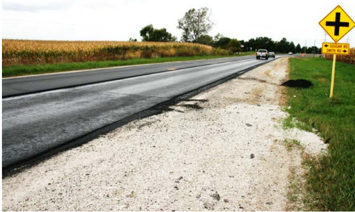
Figure 4.9. US 52 (Gougar Road to Second Street—60Y07) tack coat of level binder under traffic.
