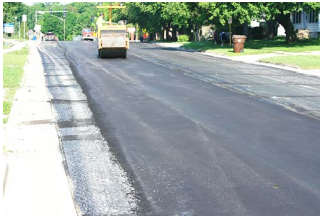
Figure 4.7. Curb-and-gutter section of Washington St. (60Y04) level binder construction and milling at gutter edge.
