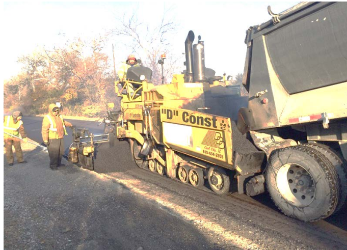
Figure 4.10. Surface course paving of rural cross-section on US 52 (US 53 to Laraway 60Y02).
