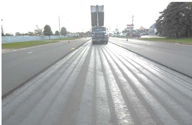
Figure 4.8. Crawford Avenue/Pulaski Road (60Y03) tack coat of level binder in center lane without traffic.
