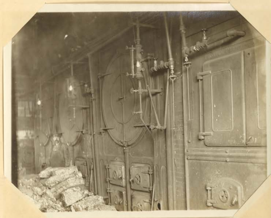
Boiler Room, Showing Method of Handling Coal.
