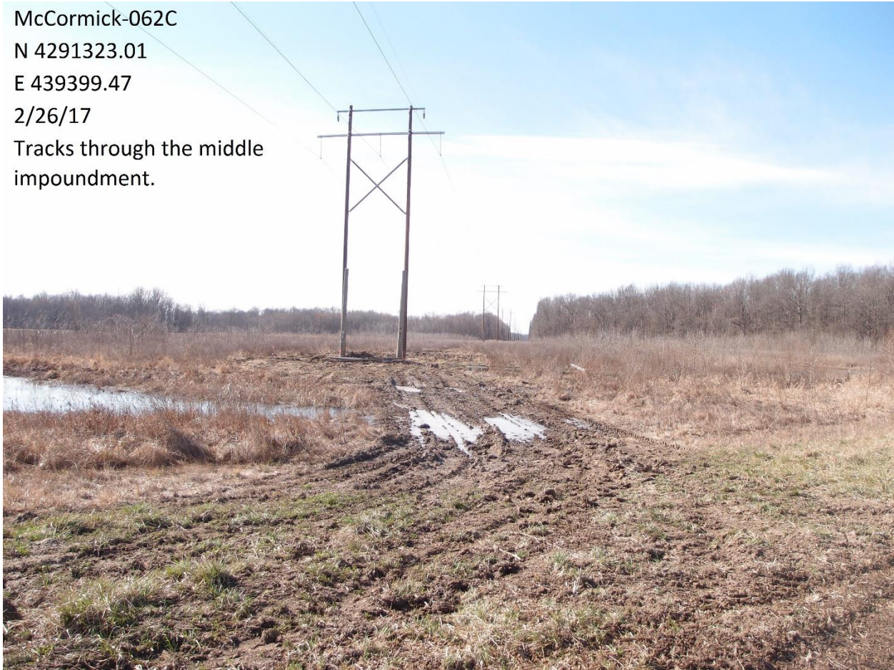
Photo 4. Southerly view of large ruts created through a wetland impoundment on the McCormick (062C) Easement in Lawrence County, Illinois. Ruts were caused from electrical crews replacing power line poles during February 2017.
