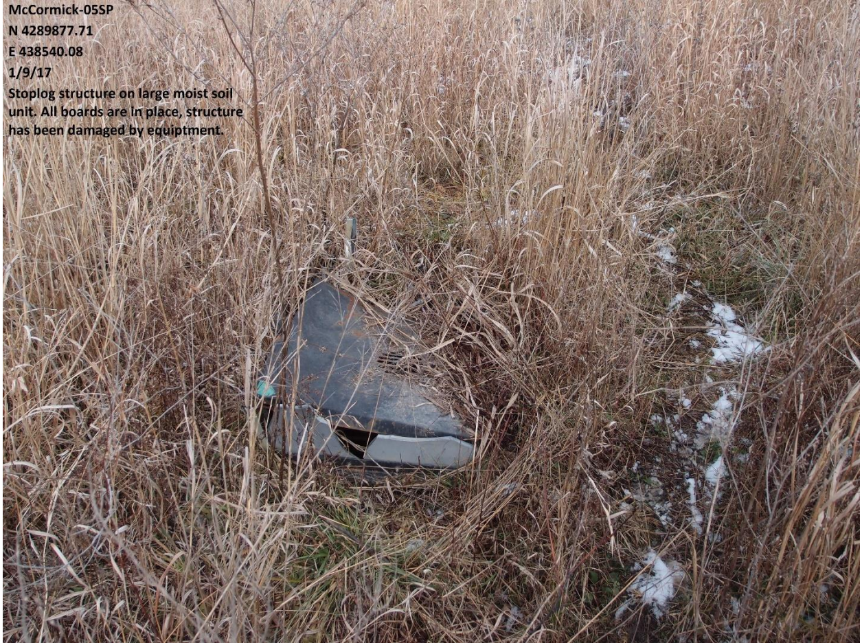
Photo 2: Cracked structure on the large emergent wetland.
