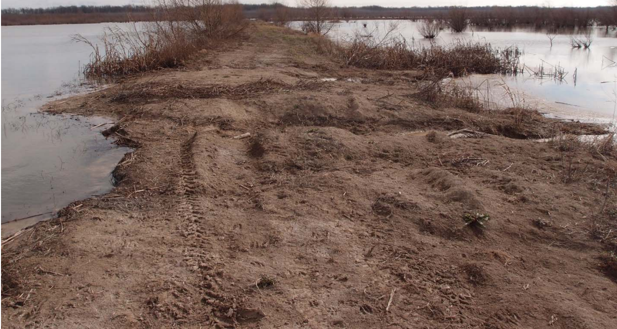
Photo 1: Damage to the levee surface from floodwaters overtopping levee surface.
