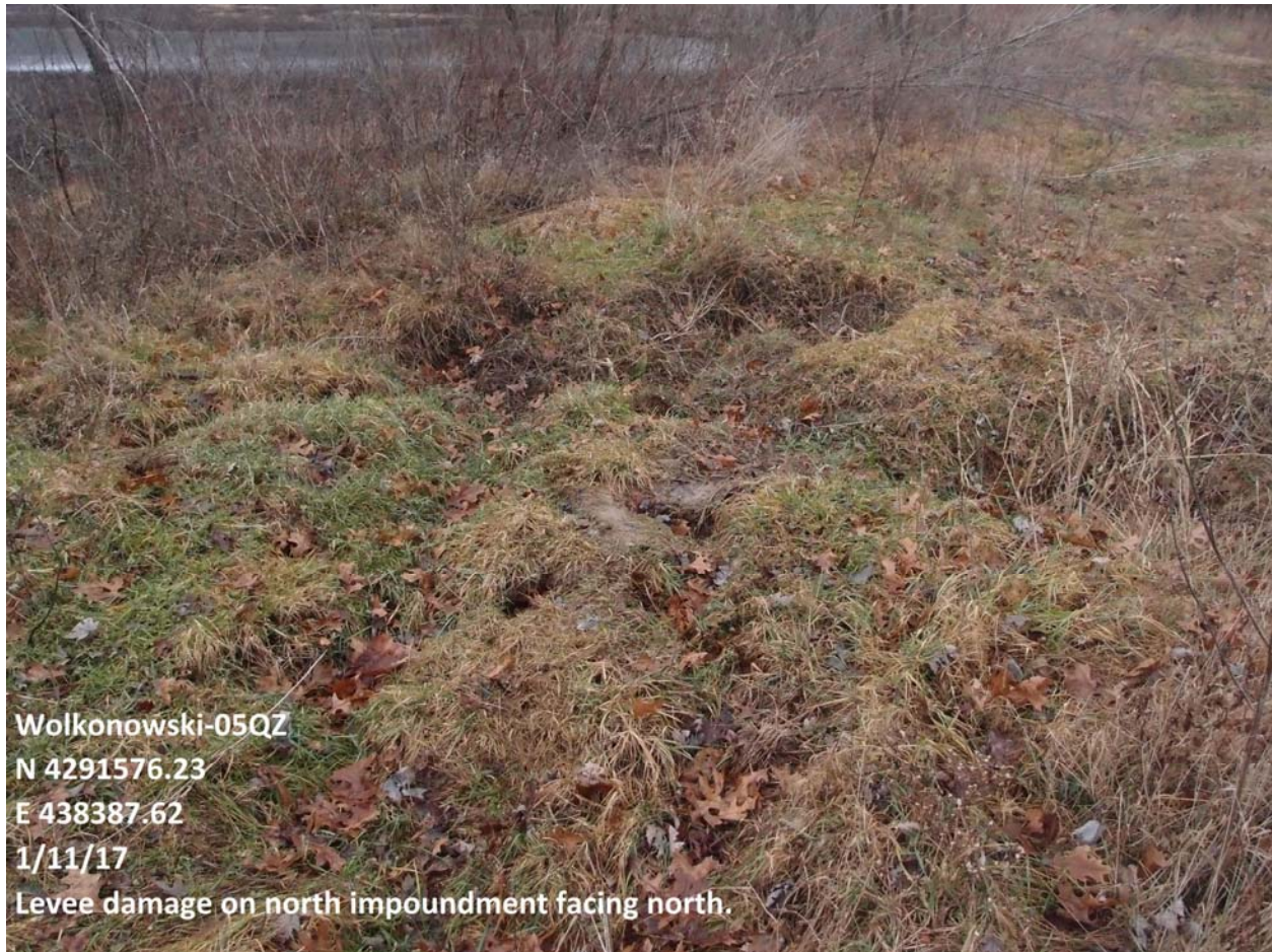
Photo 2: Large cut in levee, limiting amount of water wetland can hold.
