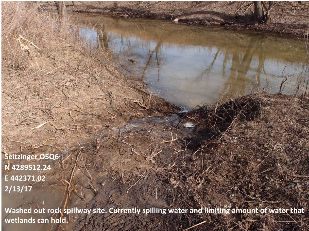
Photo 1: Eroded rock spillway site
