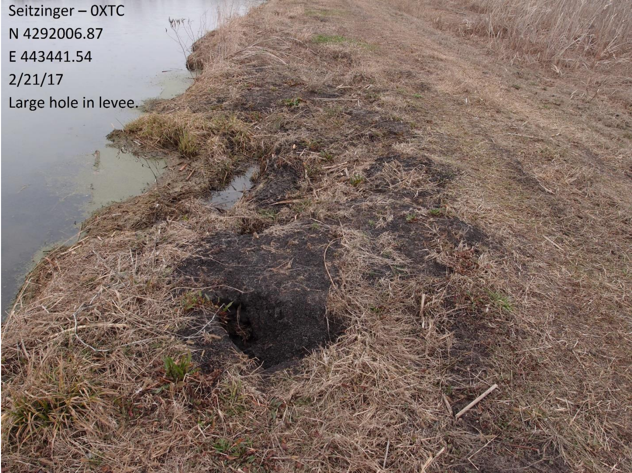
Photo 2. Levee damage from burrowing mammals on the Seitzinger OXTC Easement in Lawrence County, Illinois, during February 2017.
