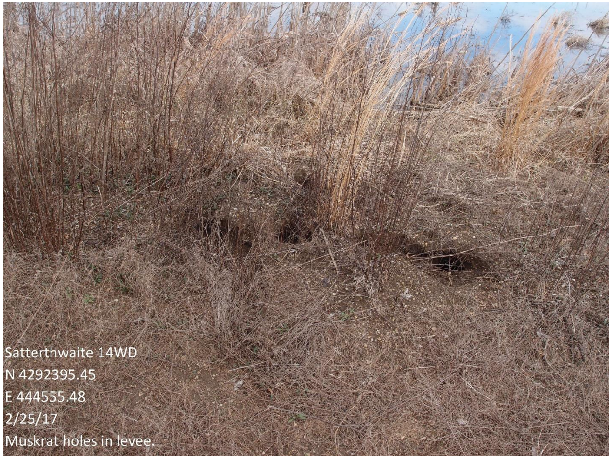
Photo 2. Damaged levee from burrowing mammals observed during the February 2017 site visit of the Satterthwaite Easement in Lawrence County, IL.
