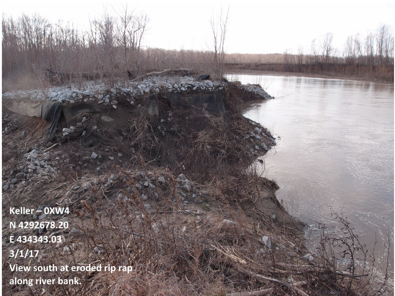
Photo 3: Rip-rap eroded from bank of the Embarrass River.
