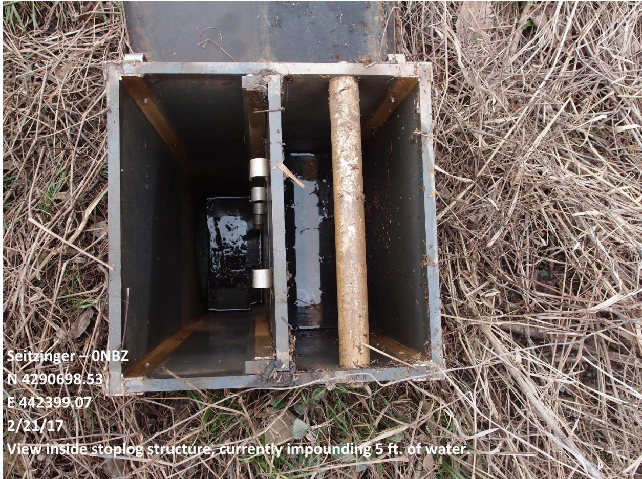
Photo 1. Stoplog structure on the Seitzinger Easement. The structure impounded water on the easement exceeding 5 ft. in depth.
