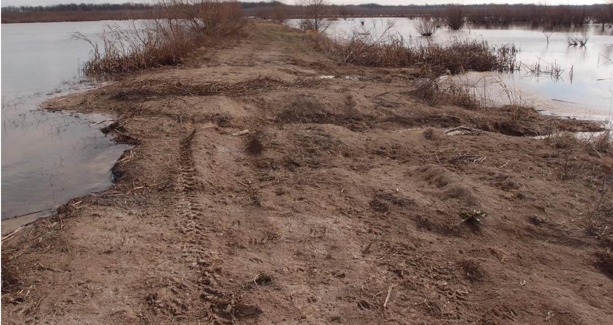
Photo 3. Easterly view of a scoured levee due to flood waters on the Bailey (05PN) Easement in Wayne County, Illinois during February 2017.
