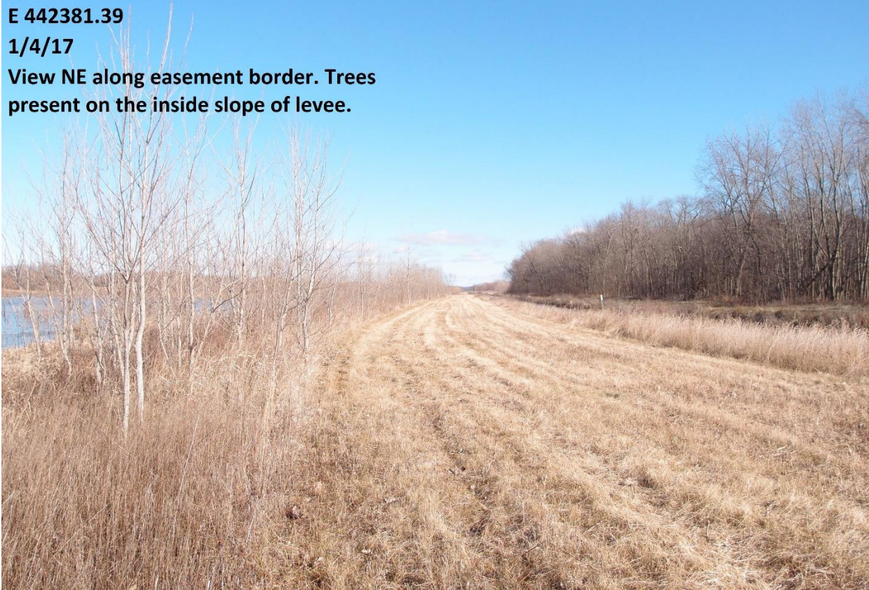
Photo 3: Woody encroachment on the inside slope of the east levee.
