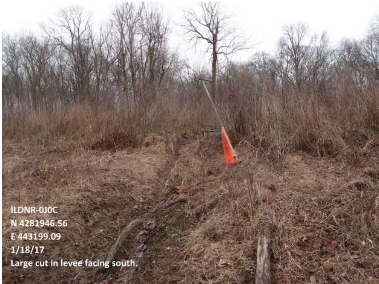
Photo 2: Southerly view of a cut in an impounding levee that influenced inundation levels within the wetland. Photo was taken on the ILDNR (0J0C) easement located in Lawrence County, IL. during January 2017.
