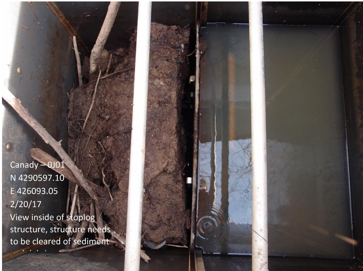
Photo 2. Example of an inoperable stoplog structure on the Canaday (0J01) Easement in Lawrence County, Illinois during February 2017.
