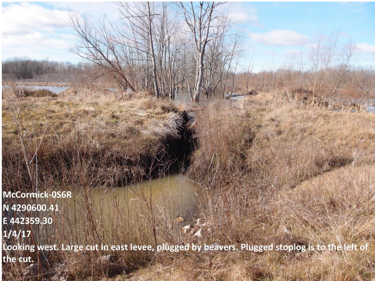
Photo 2: Westward view of a large cut in levee next to the water control structure.
