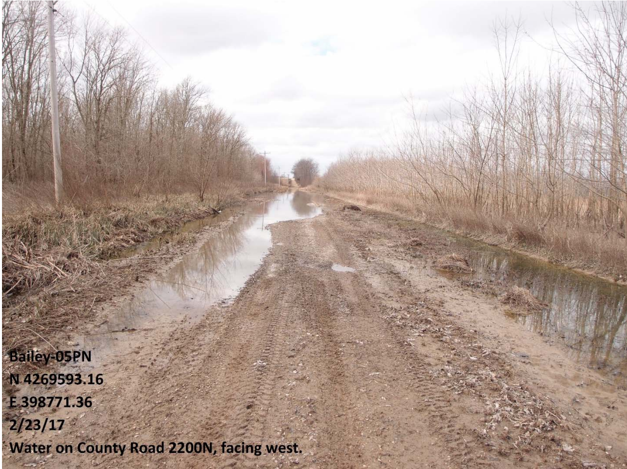
Photo 3: Flooded county road on the south side of the easement.
