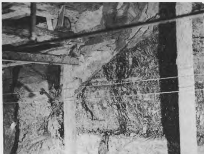
Fig. 2. - North side of south "cut-out" 4th NW entry, Peabody Coal Company No. 9, Taylorville, Illinois. The "cut-out" cuts across the coal into the underclay.
