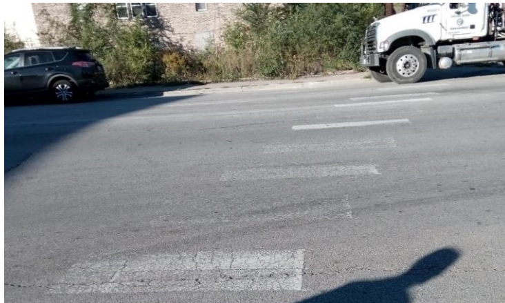
Figure E-69. Crosswalk markings at intersection of S. Pulaski Rd. and Folk St.
