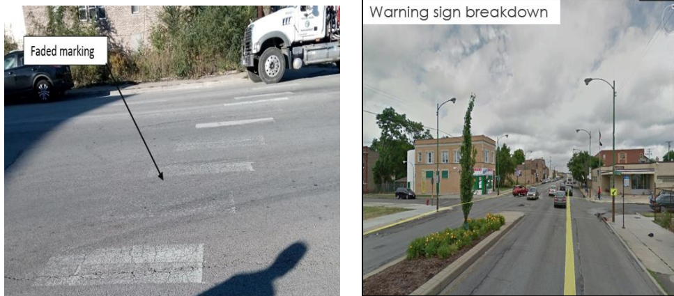
Figure 34. Example of lack of maintenance for crosswalk markings and signs.
