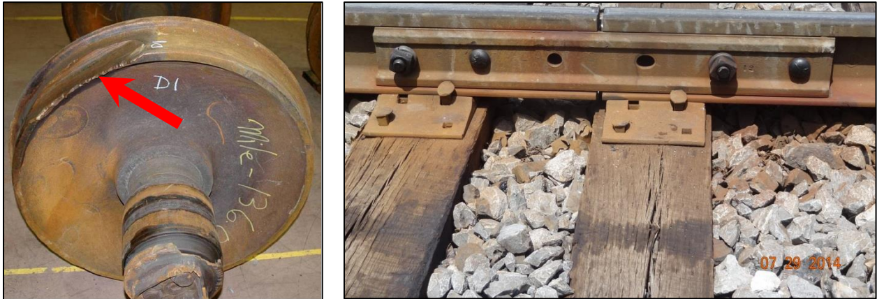
Figure 2.38: (a) Photograph of wheel flat (TSBC, 2007) and rail joint with joint bar.
