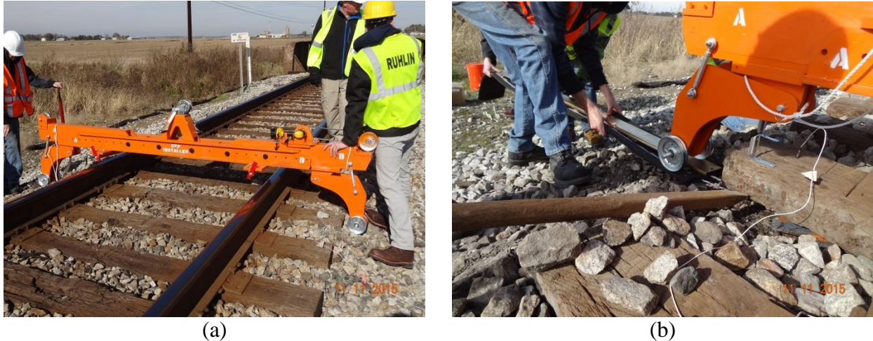
Figure 6.19: Photographs of (a) the HTS installer on track and (b) inserting UTP underneath a timber tie in track.
