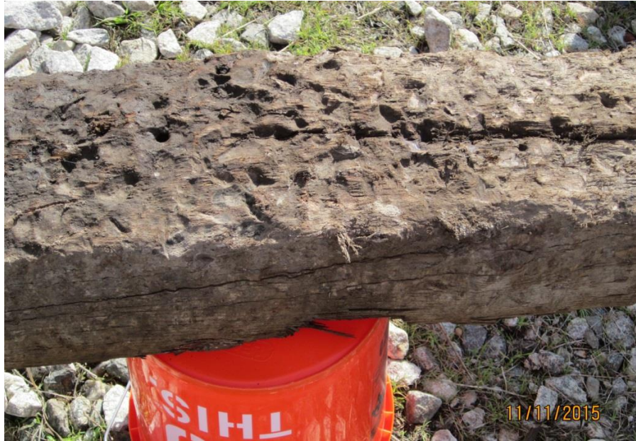
Figure 2.17: Photographs of indented ties at the tie-ballast interface.
