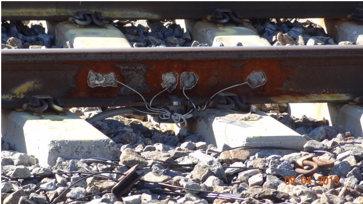
Figure 3.8: Photograph showing two strain gauges in crib area for vertical wheel load and two strain gauges above the tie for tie reaction.
