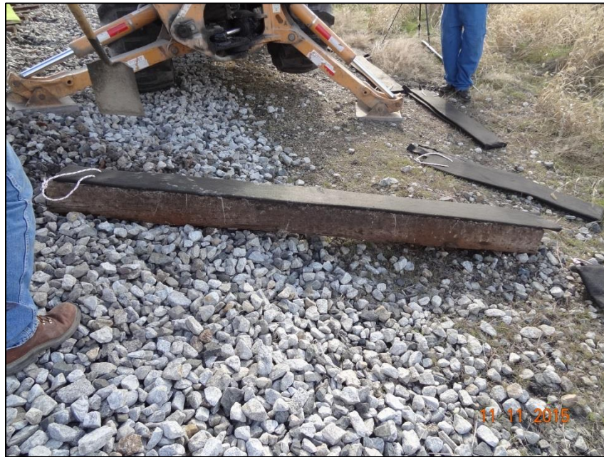
Figure 6.11: Photograph of under-tie pad (UTP) on a timber tie.
