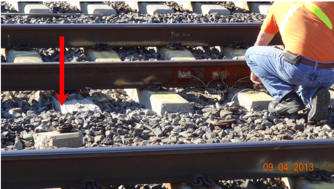
Figure 3.55: Photograph of damaged tie to the left of the MDD instrumentation location (see red arrow) at Madison (12 ft.) on 4 September 2013.
