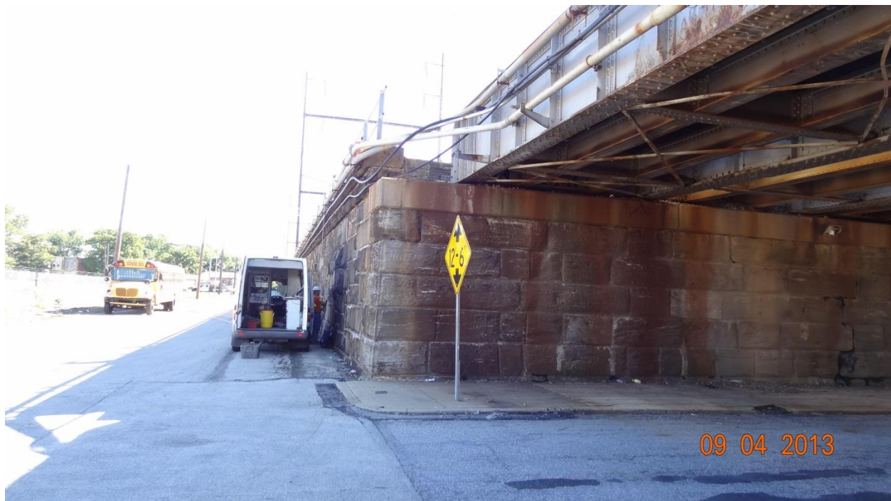
Figure 3.9: Photograph of masonry walls at Upland Avenue below the Upland (15 ft) MDD location with Mike Tomas collecting MDD cables.
