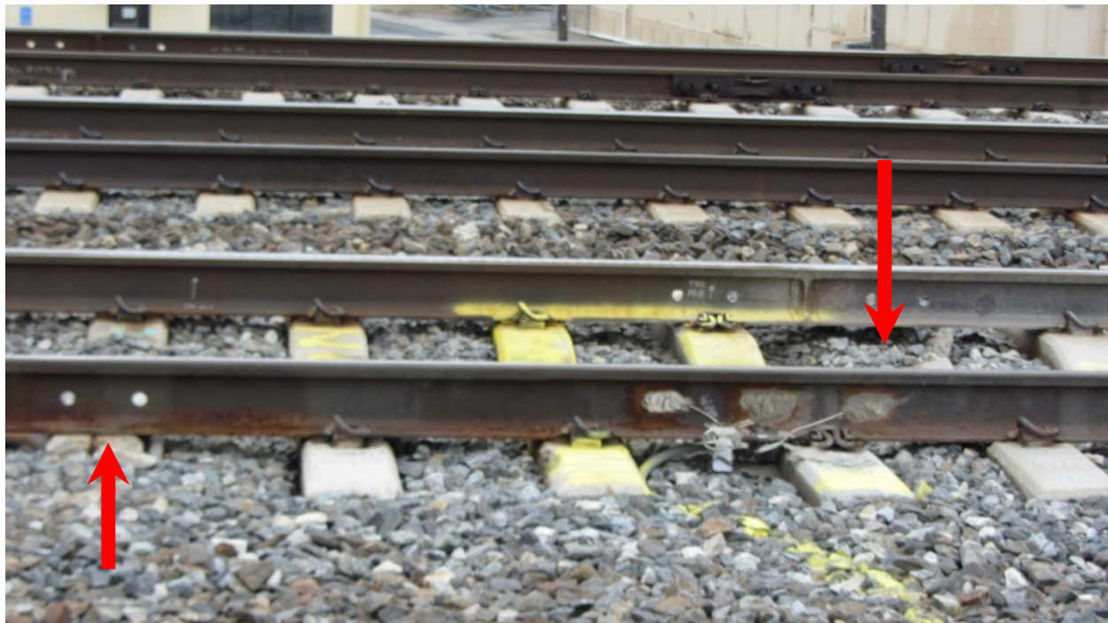
Figure 3.56: Photo of two damaged ties near the Upland (15 ft.) instrumentation location (see red arrows). Damaged ties are three ties to the left and one tie to the right of the instrumented tie which have been replaced as of July 2013. (Photo taken by Deb Mishra.)
