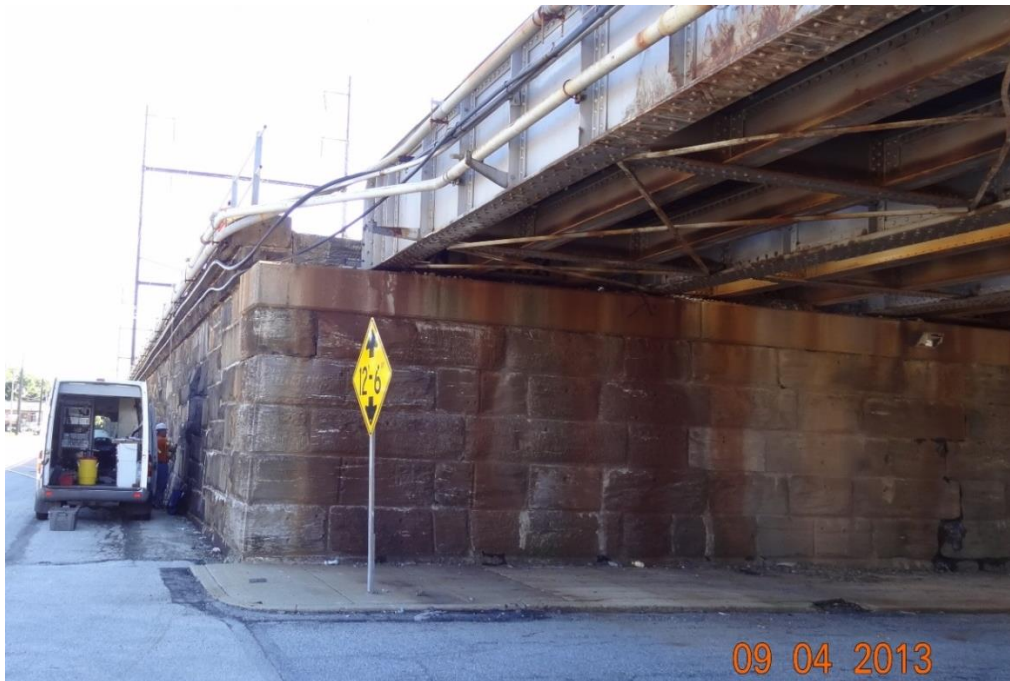
Figure 5.38: Photograph of masonry walls at Upland Avenue below the Upland (15 ft.) instrumentation location looking north with Mike Tomas' truck adjacent to wall with MDD location on Track #3 above the white truck.
