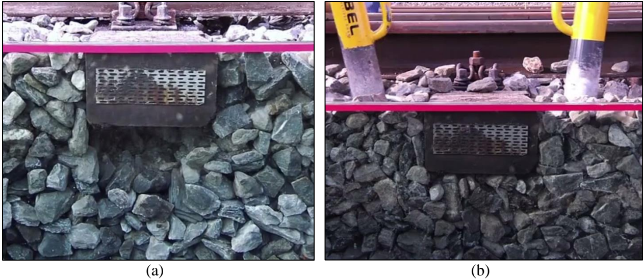
Figure 6.15: Photographs of tie and underlying ballast (a) before and (b) after tamping (courtesy of Robel Company).
