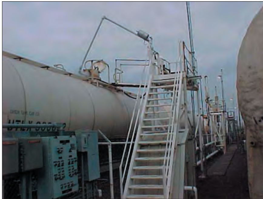
Figure 6.1. Rail towers for unloading CO 2 from railcars
