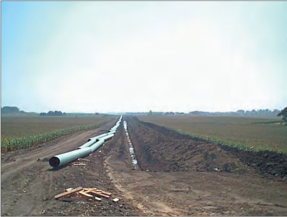
Figure C1.18. Pipe is ready for pipe gang—the pipe is strung on skids, the ditch is complete, and the ditch spoil is segregated from topsoil
