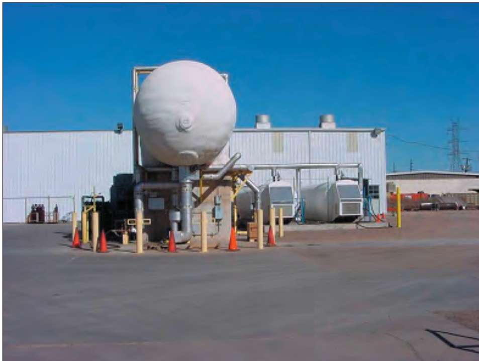
Figure 5.1. Secondary storage tanks
