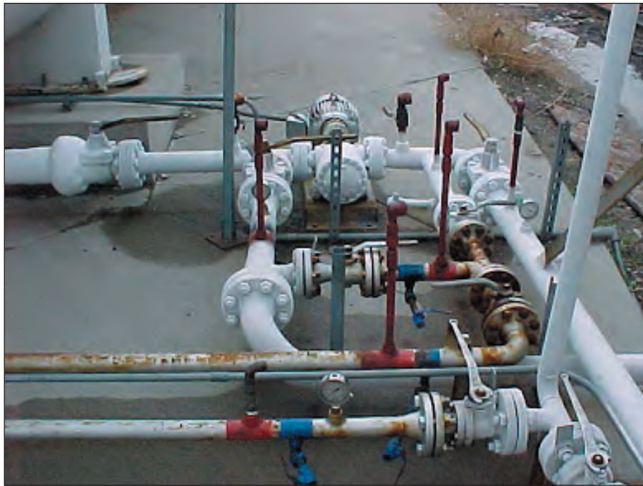
Figure 6.3. Typical CO 2 injection skid
