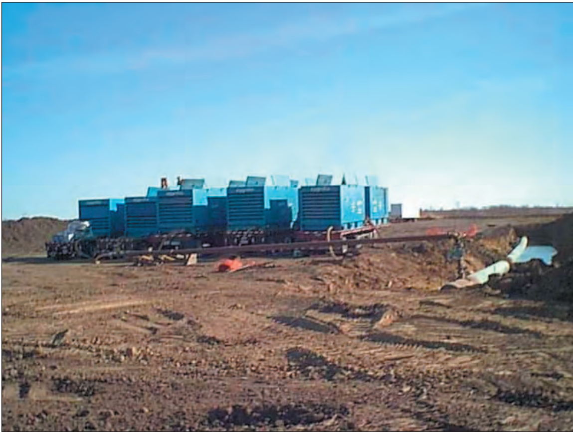
Figure C1.37. Bank of air compressors set up for dewatering of the test segment
