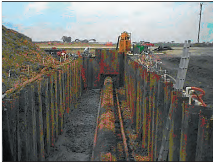
Figure 6.9. Road bore in a sandy area with high groundwater showing required sheet pile and ground dewatering systems
