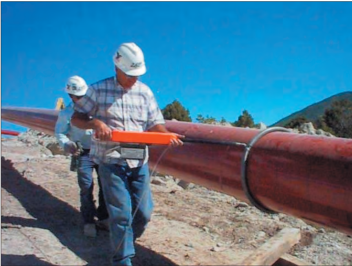
Figure C1.25. Jeeping for pipe coating defects
