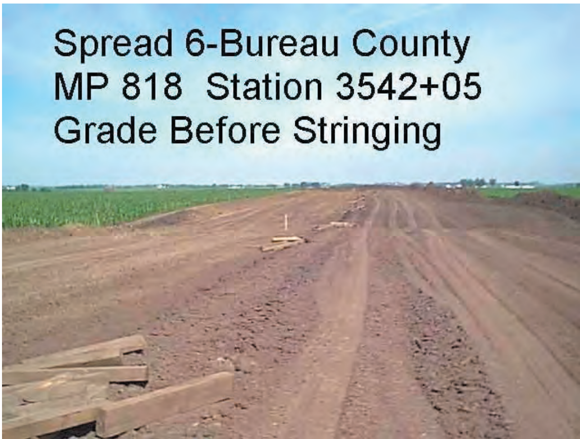
Figure C1.5. Completed grading. Note that the skids stringing, pipeline centerline stakes, and topsoil are stockpiled at the edge of the right-of-way
