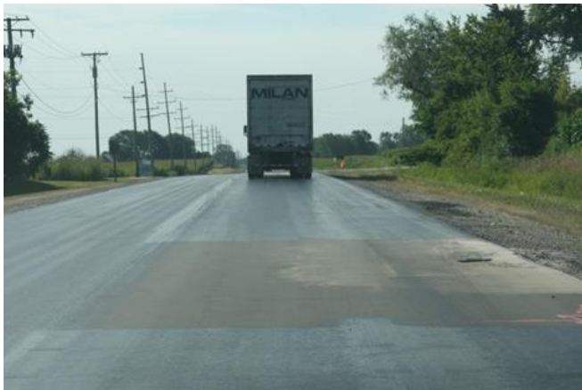
Figure 28. Edge distress of US 52 looking south near Sta. 42+00 looking north.
