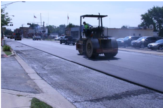
Figure 34. Level binder roller train; primed and milled parking area with filled joint/crack near Sta. 84+00 westbound lane looking south.
