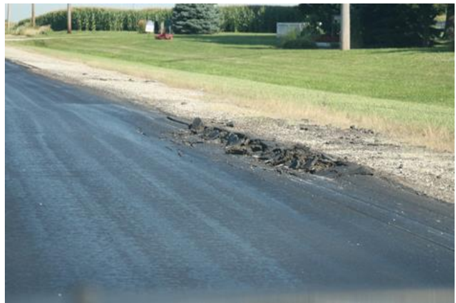
Figure 27. Edge of pavement distress on westbound US 52 near Sta. 77+00.
