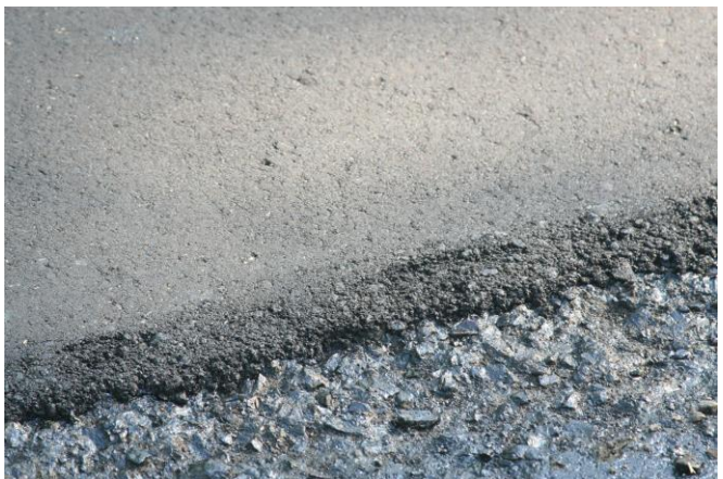
Figure 15. Segment 2 (Peale to US 30) showing 1 ft milled pavement to be covered with surface course.
