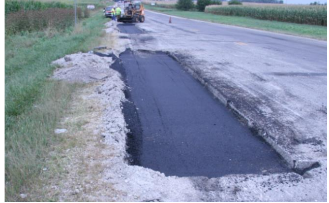
Figure 33. US 52 patch near Sta. 36+00 eastbound lane looking north.
