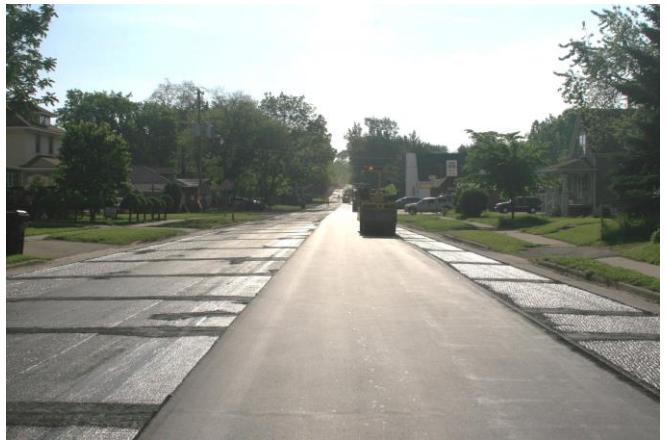
Figure 13. Segment 1 (Briggs to Peale) level binder placed with luted tapered edge (right side) to edge to milled concrete.
