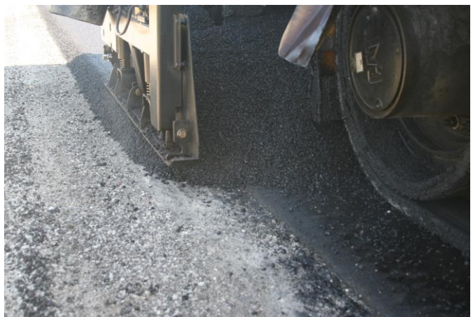
Figure 25. Surface course installation showing level course, lip between level and cold-milled surface, and surface course installation.
