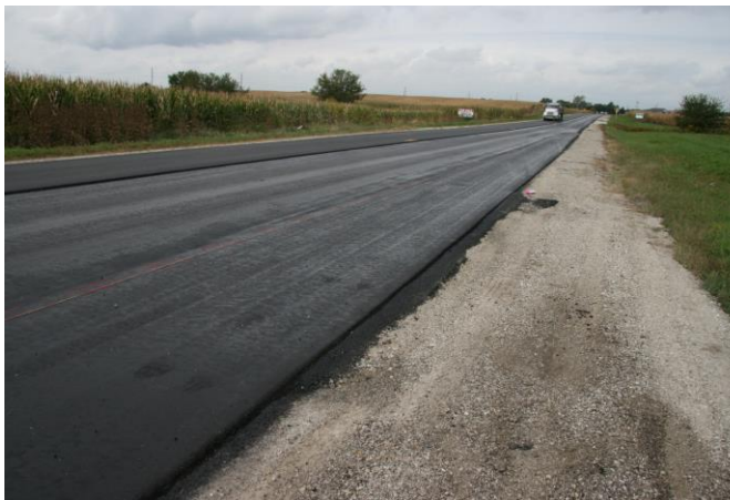
Figure 38. Near Sta. 36+00 looking north with surface placed eastbound. Note level binder placed 1 ft less than lane width.
