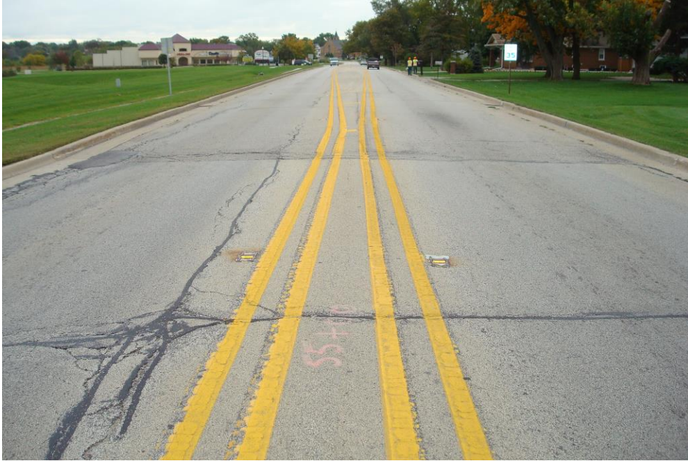
Figure 7. US 52–Gougar Road to north of Second Street near Station 55+00 looking south.
