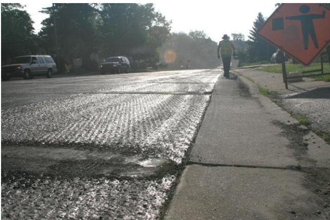
Figure 8. Segment 1 (Briggs to Peale) cold-milled pavement looking east.
