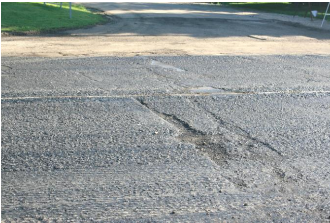
Figure 12. Segment 2 (Peale to US 30) possible area needing patching.
