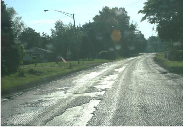
Figure 10. Segment 2 (Peale to US 30) cold-milled pavement looking east.
