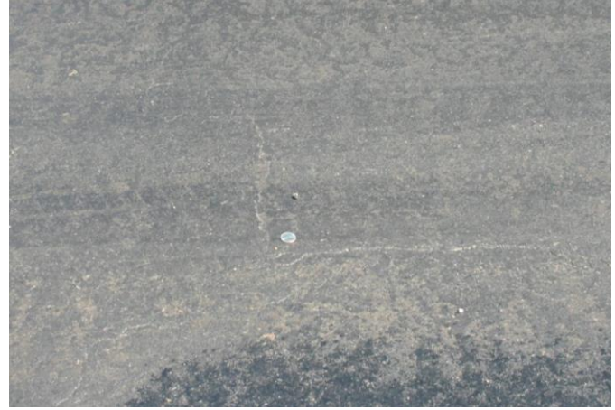
Figure 17. Segment 2 (Peale to US 30). Longitudinal and transverse cracks in newly placed level binder east of NE Circle Drive in westbound lane outer wheel path.
