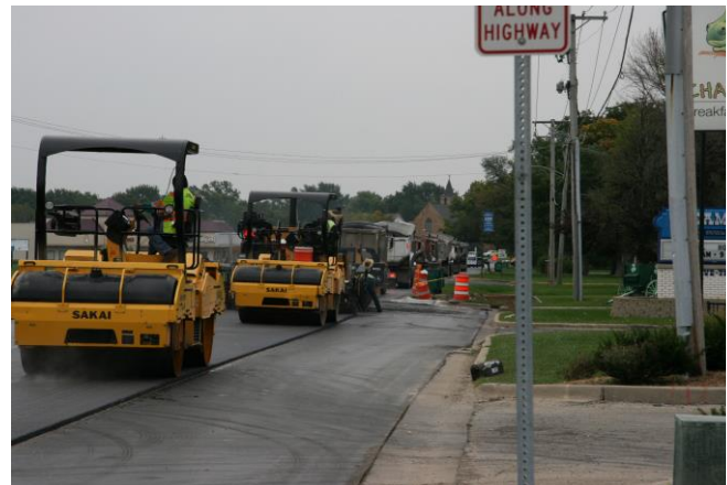
Figure 39. Paving train of surface in eastbound lanes just south of Manhattan Road.
