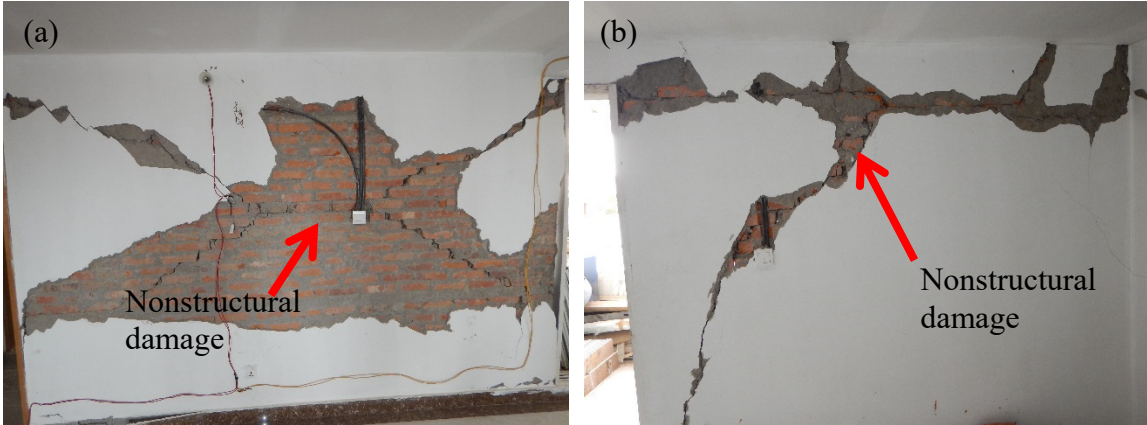
Figure 3.30 Silver City Apartment Complex – interior non-structural masonry wall damage in east-west direction.
