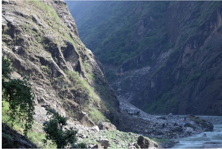
Figure 2.13 Rockfall upstream of the hydropower project (after Hashash et al. 2015).
