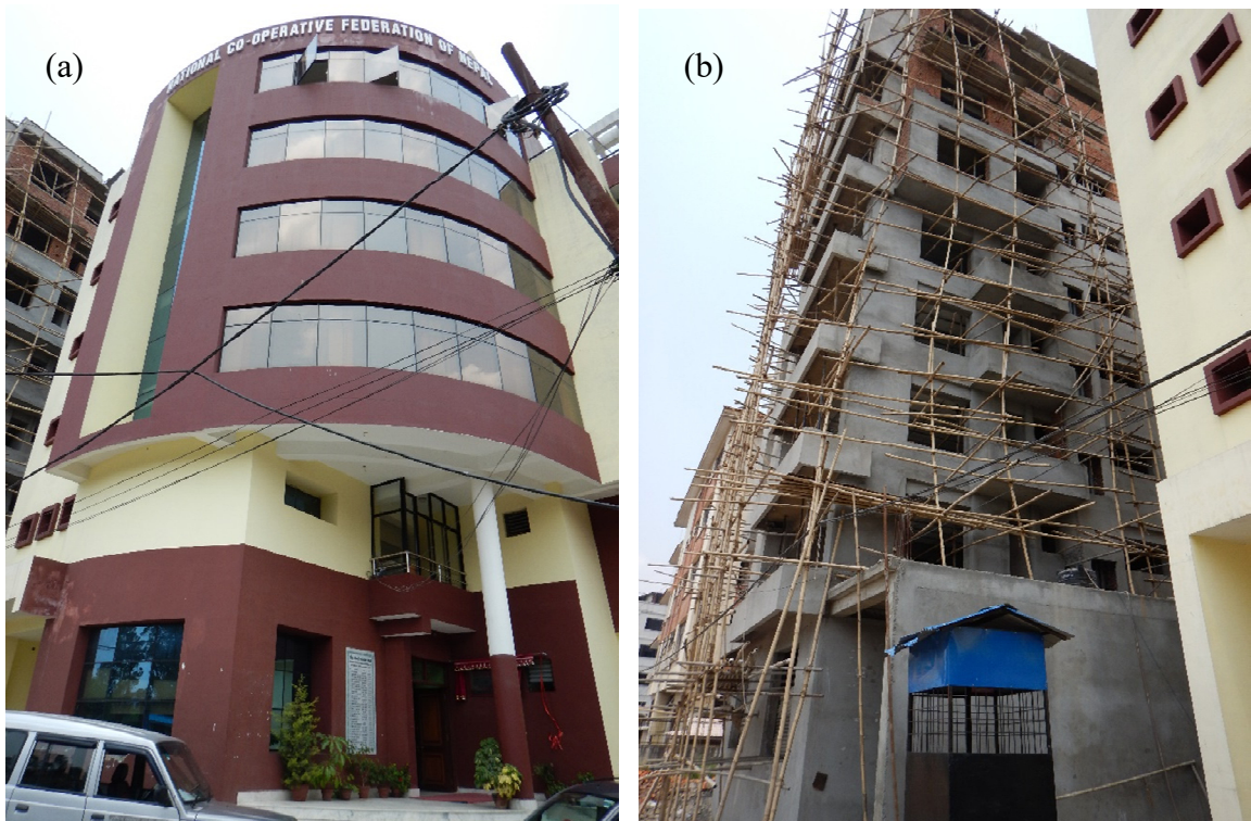
Figure 3.12 New buildings designed by Pumori Engineers: (a) occupied 6-story building; (b) 8-story building under construction.
