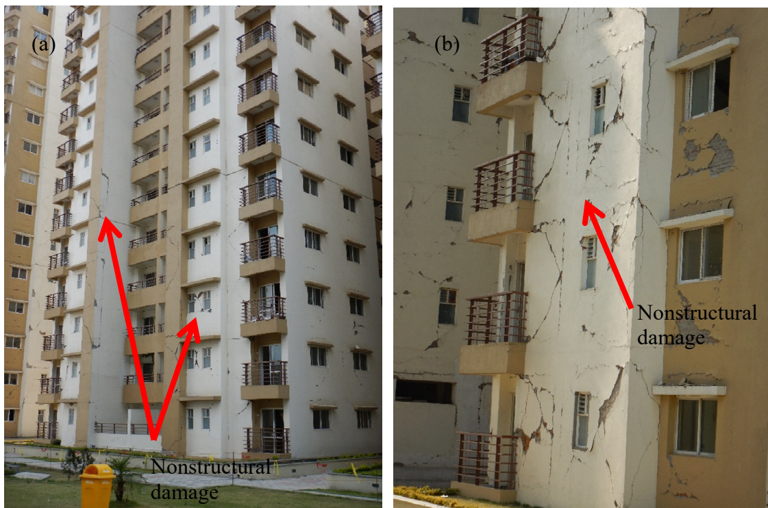
Figure 3.24 Cityscape – moderate non-structural damage: (a) overall view; (b) detail view.
