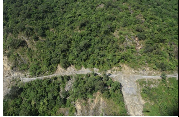
Figure 2.8 Gabion retaining walls that did not perform well along the Charikot-Lamabagar Road.
