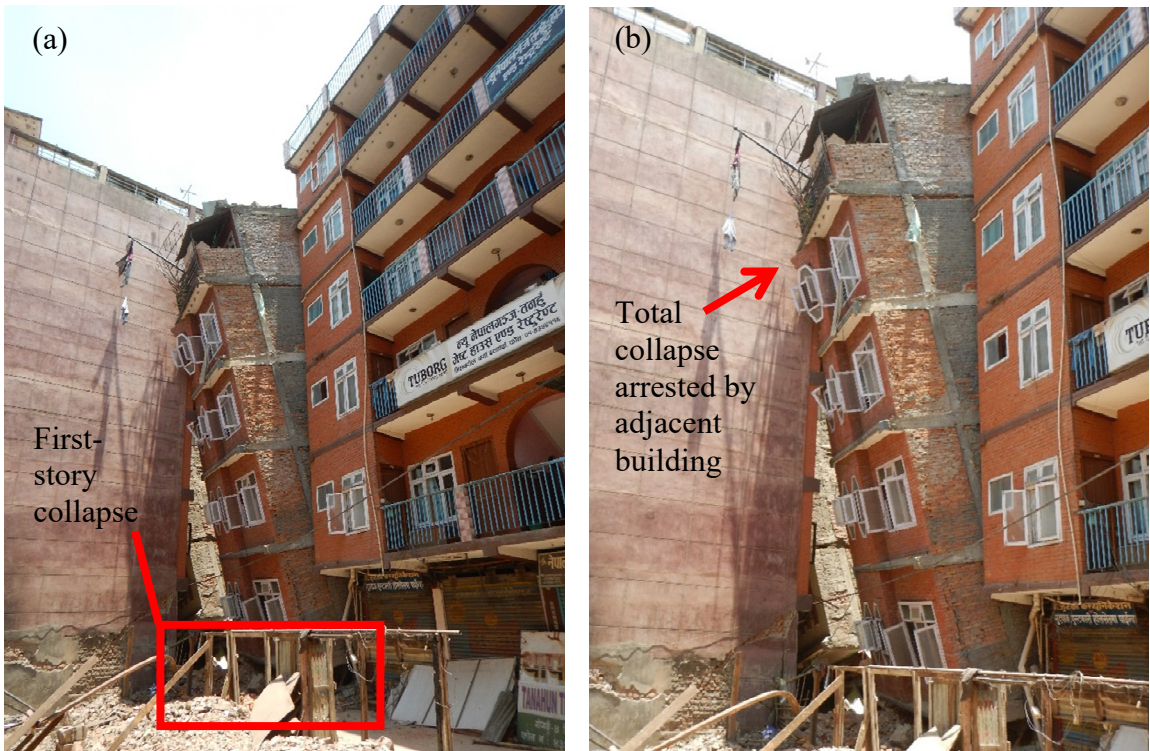
Figure 3.2 RC frame building with first-story collapse; Balaju, Kathmandu: (a) overall view showing first story collapse; (b) zoomed-in view showing contact with adjacent building.
