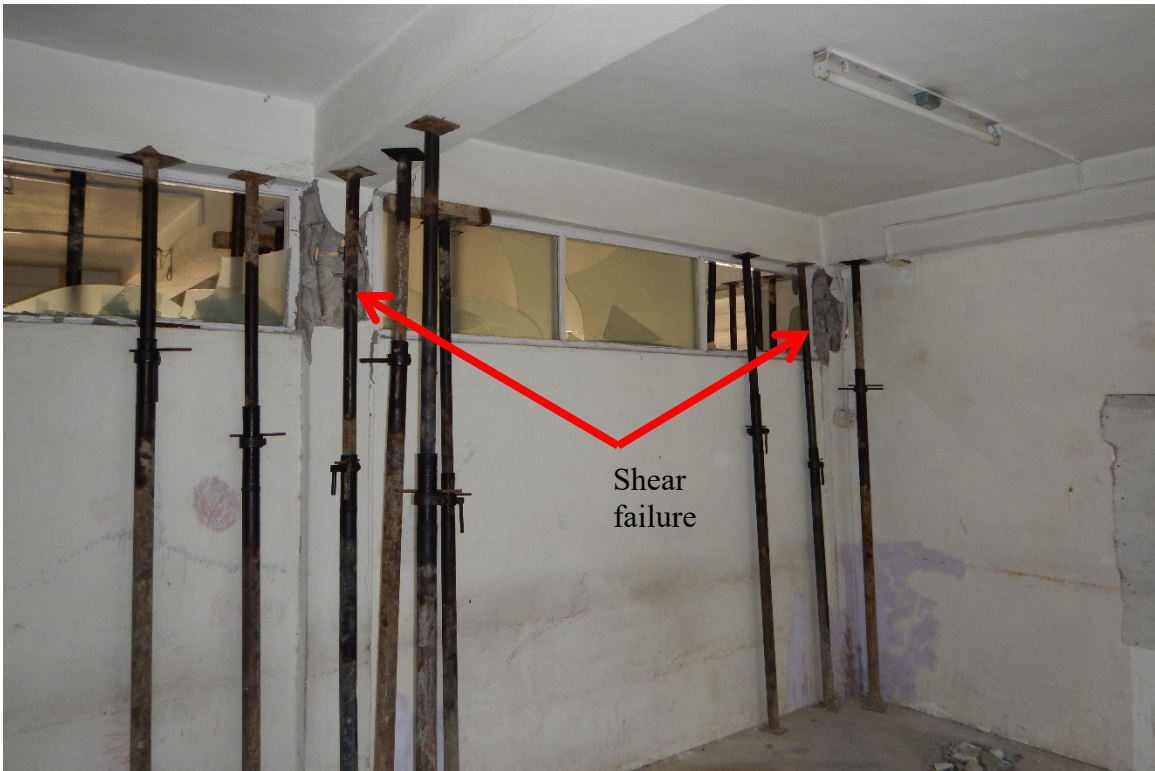
Figure 3.20 Kathmandu Engineering College Block C Building – short column shear failure.
