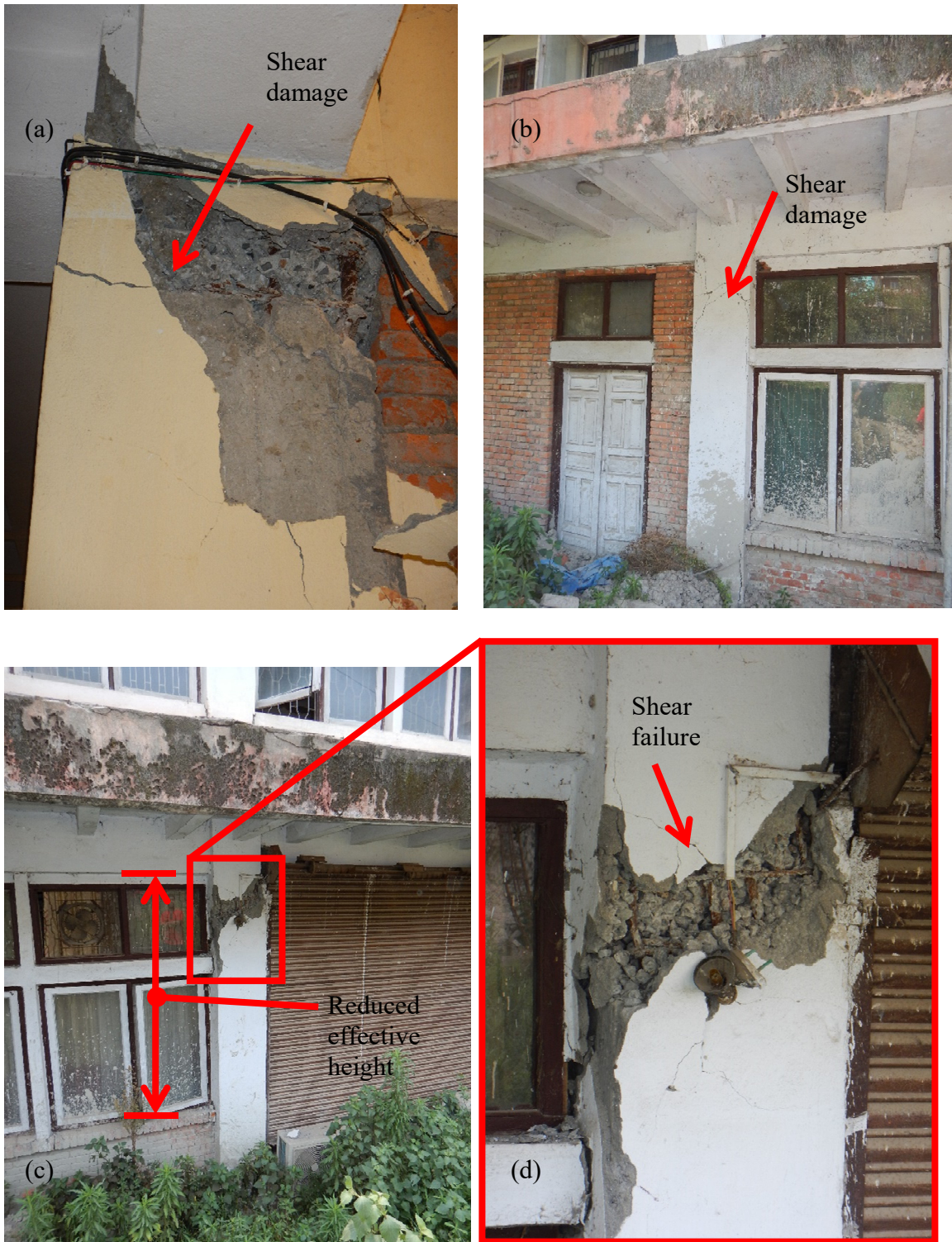
Figure 3.16 Central Fisheries Building – column shear damage at top of first story: (a) interior; (b) exterior; (c) exterior overall; (d) exterior close-up.
