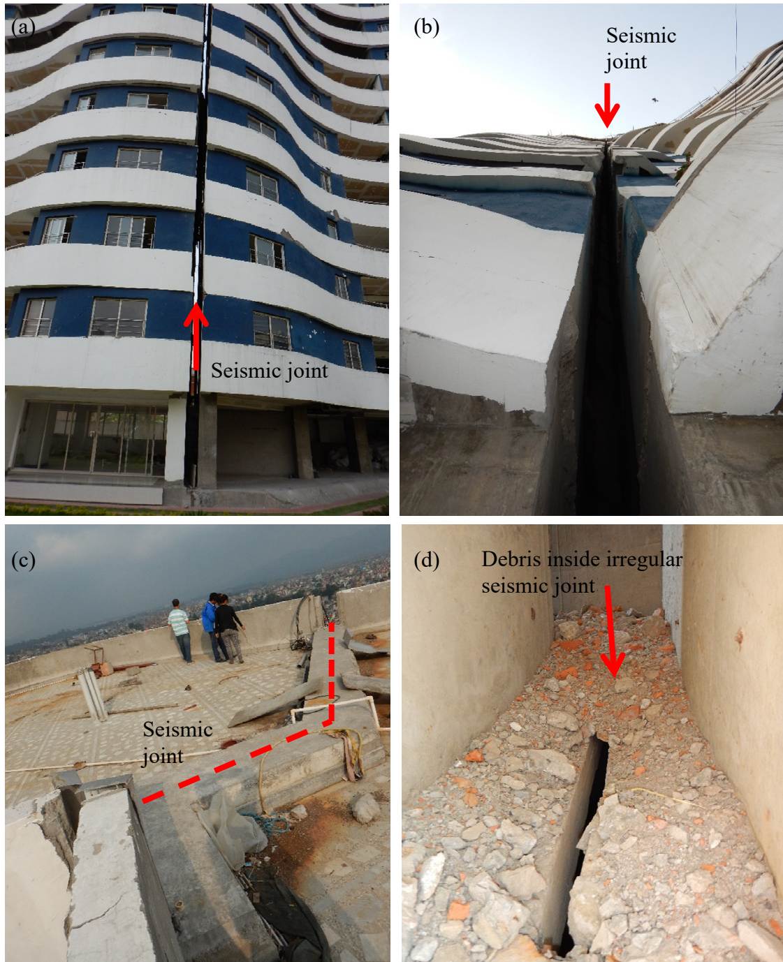
Figure 3.29 Silver City Apartment Complex – seismic joints: (a) south view of west joint, straight; (b) south view of east joint, irregular; (c) top view of east joint, irregular; (d) interior view of east joint, irregular.
