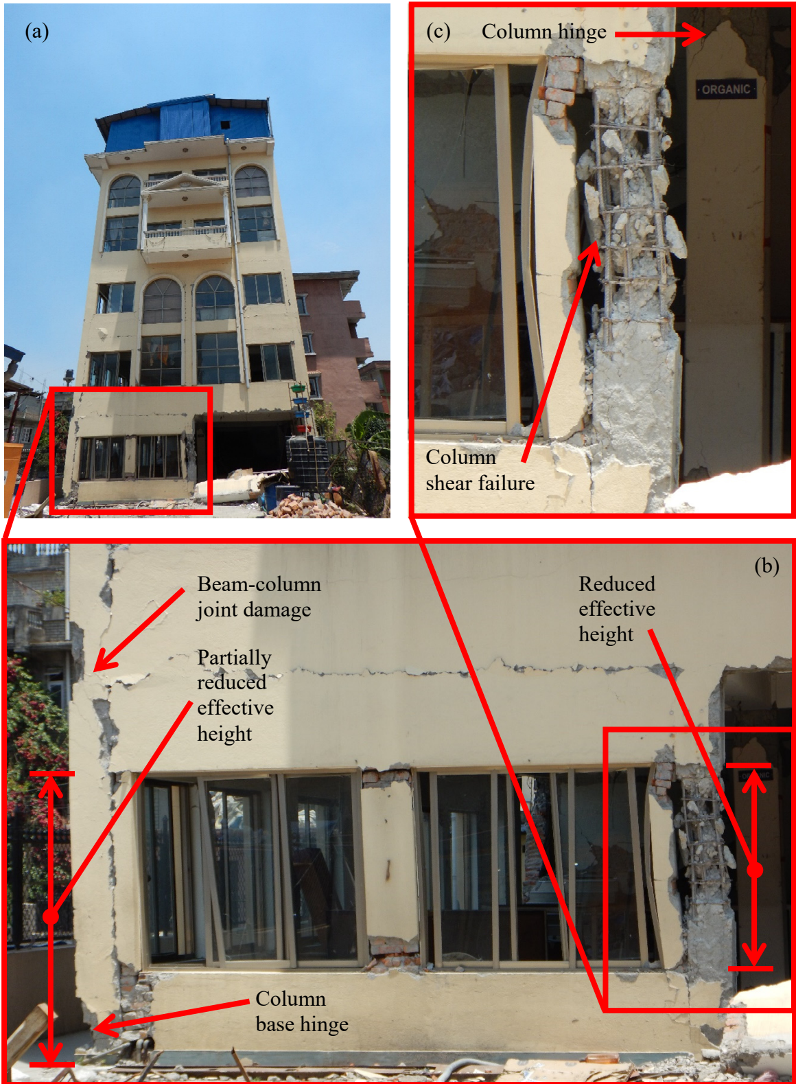
Figure 3.5 RC frame building with severe damage, but no collapse; Balaju, Kathmandu: (a) overall building view showing soft / weak first story due to drive-in bay; (b) zoomed-in view of partial first story; (c) zoomed-in view of column with shear failure.
