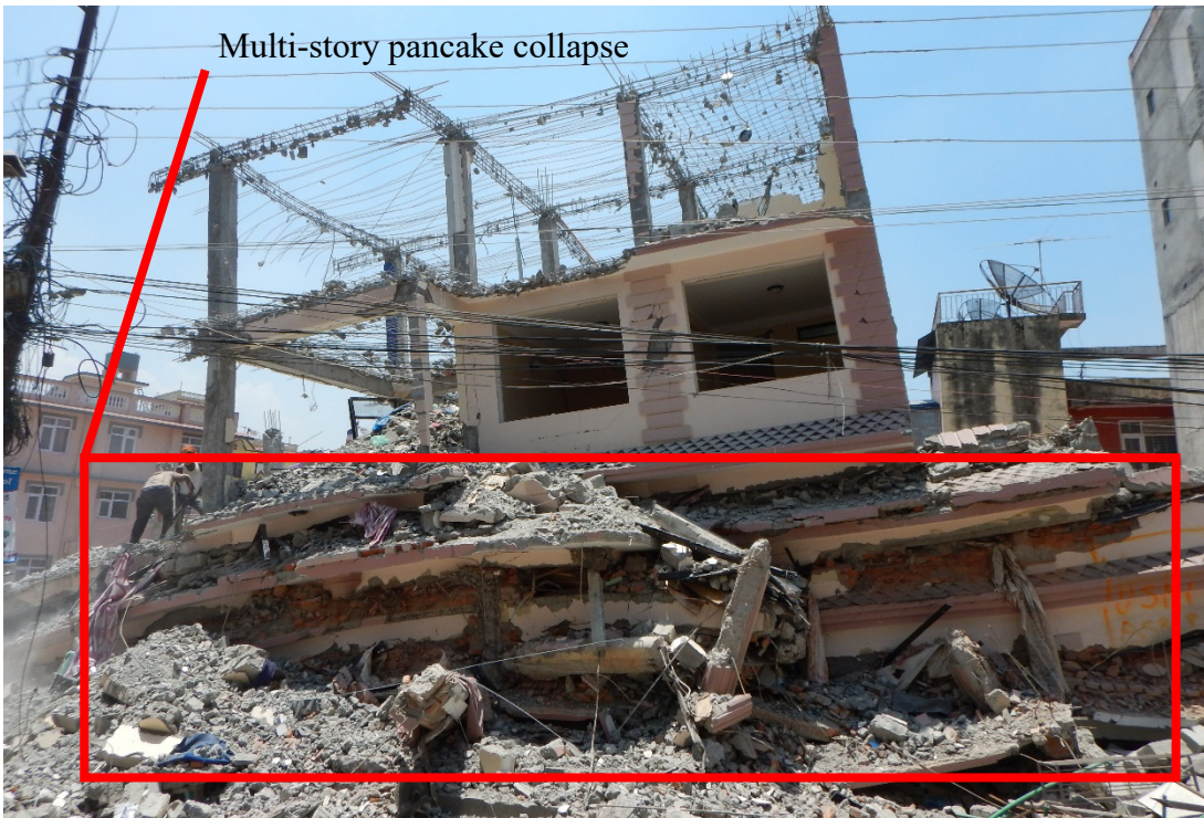
Figure 4.3 RC frame building with multi-story pancake collapse; Balaju, Kathmandu.
