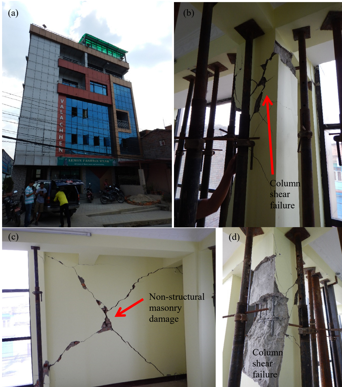
Figure 3.7 Valachhen Building, RC frame with structural and non-structural damage: (a) exterior elevation view; (b) column shear failure; (c) nonstructural masonry damage; (d) column shear failure.
