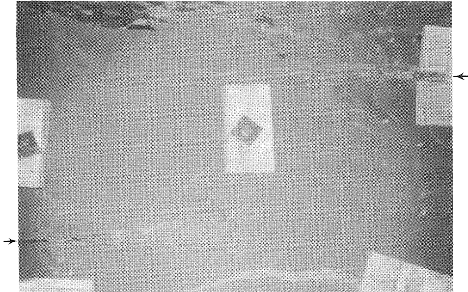
Figure 15. "Worm's-eye view" of discontinuous shear fractures in Energy Shale in the roof of Orient No. 6 Mine.
